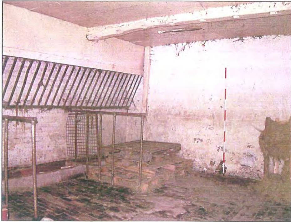
Plate 53: Southern section, north stable with feeding trough and hayrack, brick floor and drain
