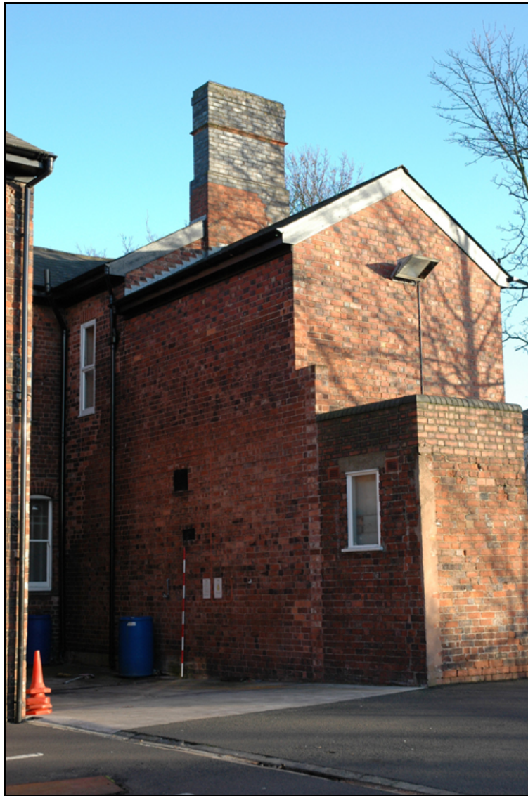
Figure 22: Chimneystack, partly built in wrong colour brick
