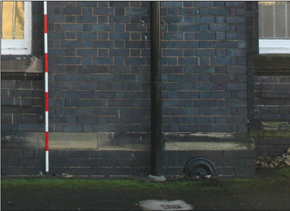
Figure 17: Buried tie rod
