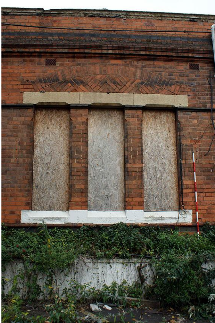
Plate 12: Building 6 triplet window with chamfered mullions and herring bone brickwork with relieving arch
