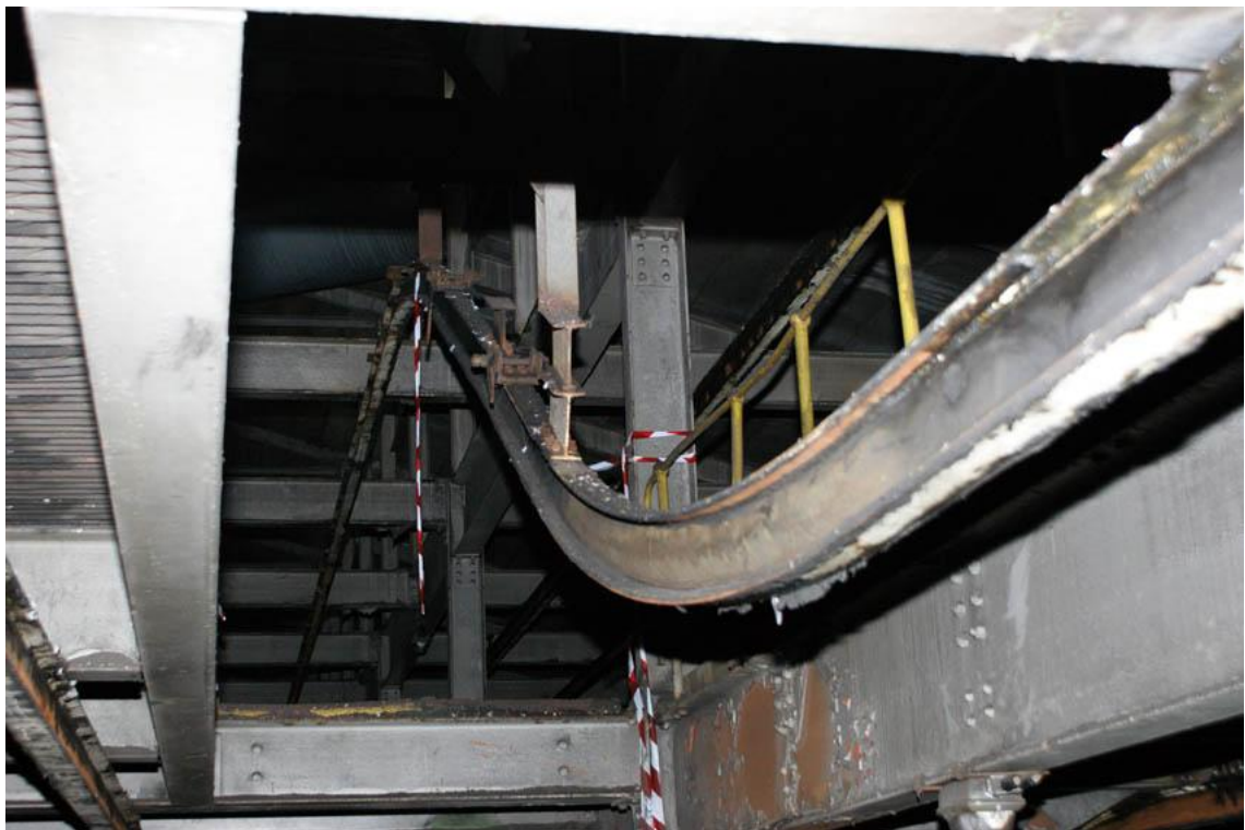
Plate 38: Travelling rail system between floors within maintenance building
