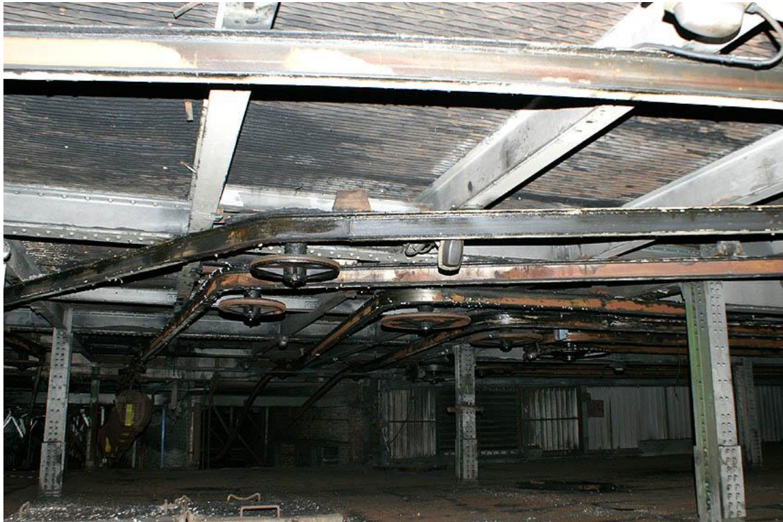
Plate 37: Travelling rail system for buckets within maintenance building
