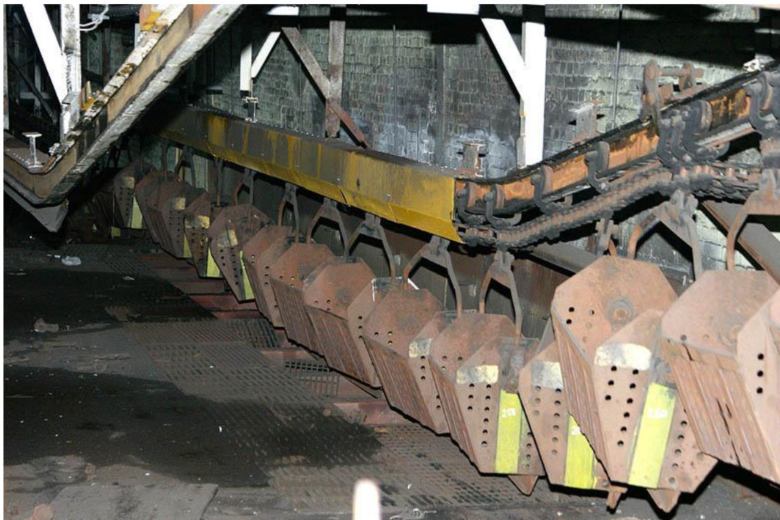
Plate 36: Buckets on No. 7 mould line within maintenance building
