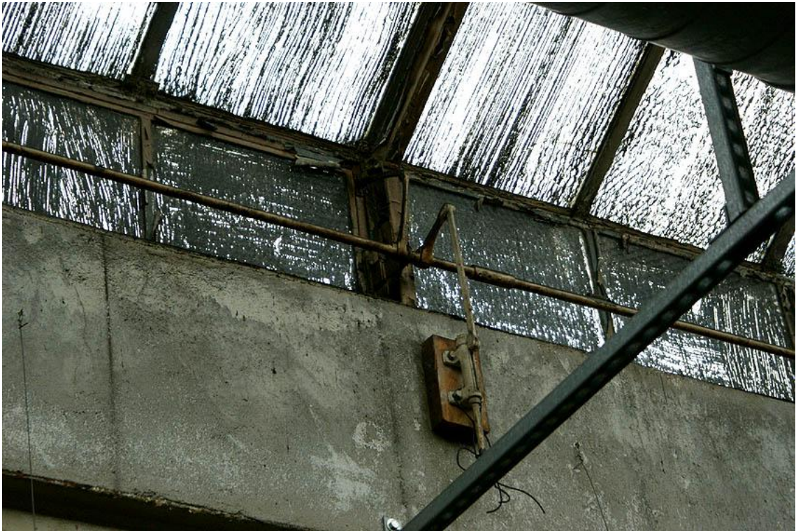
Plate 7: Skylight openers in building 5
