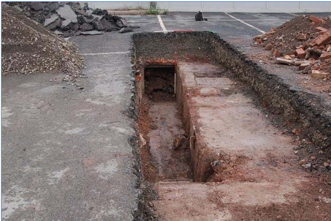
Plate 4 Trench 2 looking North showing modern 20 th Century structure and truncation by a service trench to the north.
