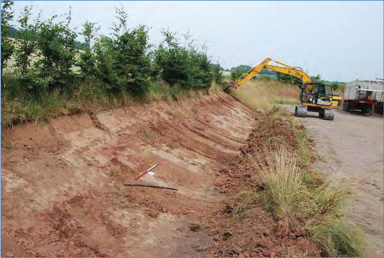
Plate 7 Soil profile of western bank exposed showing modern disused water pipe trench. View north-west
