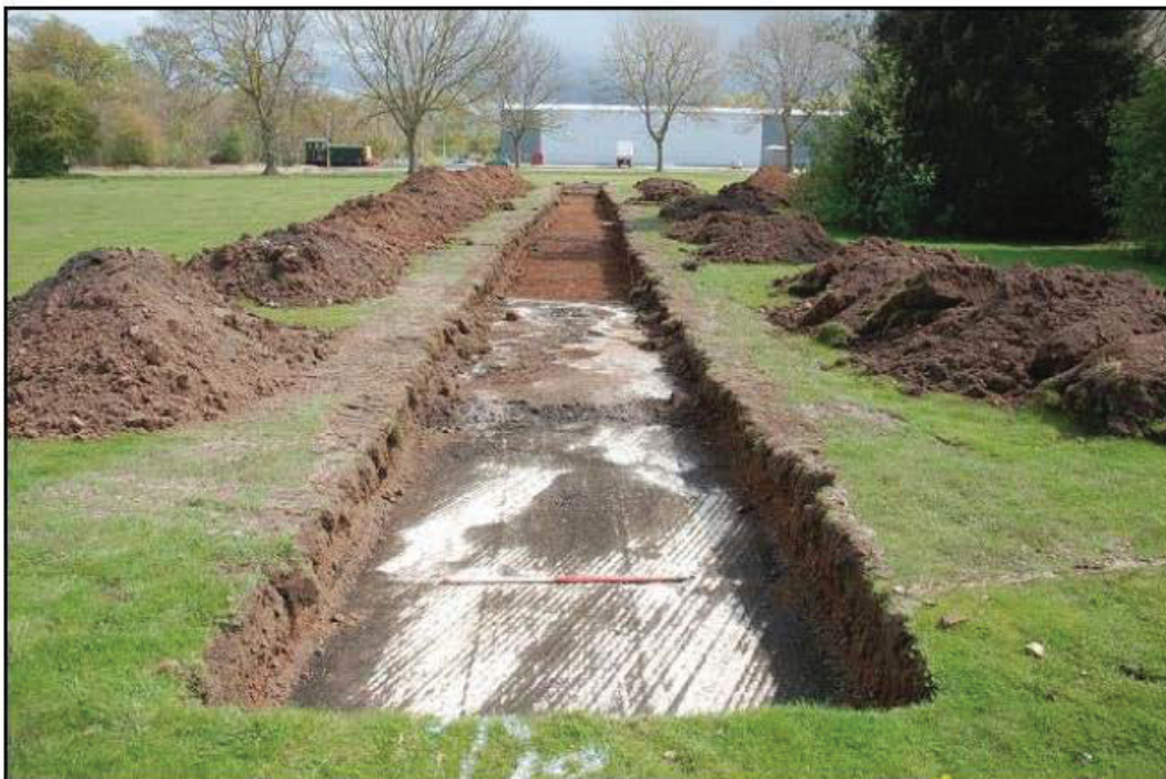
Plate 18 Trench 12 after excavation showing modern concrete slab and made ground, looking east
