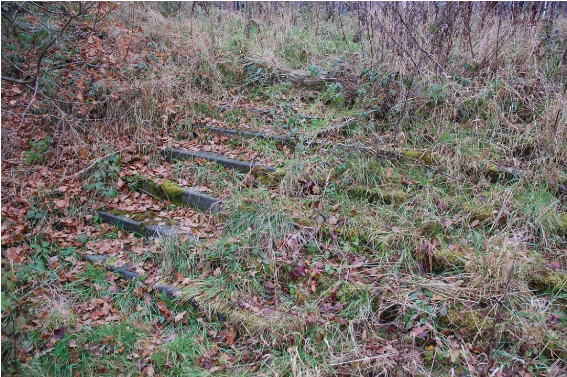
Plate 25: Condition of steps onto garden terrace by hall
