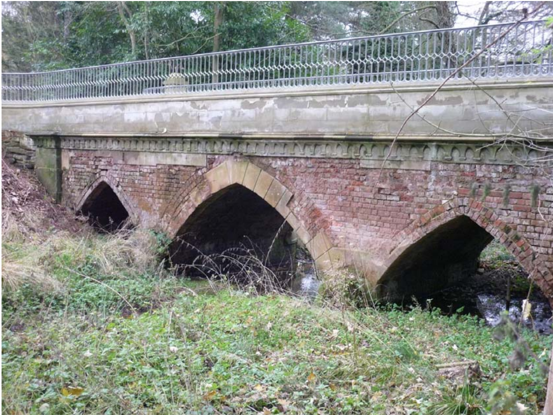
Plate 10: Current condition of Sutton's Bridge
