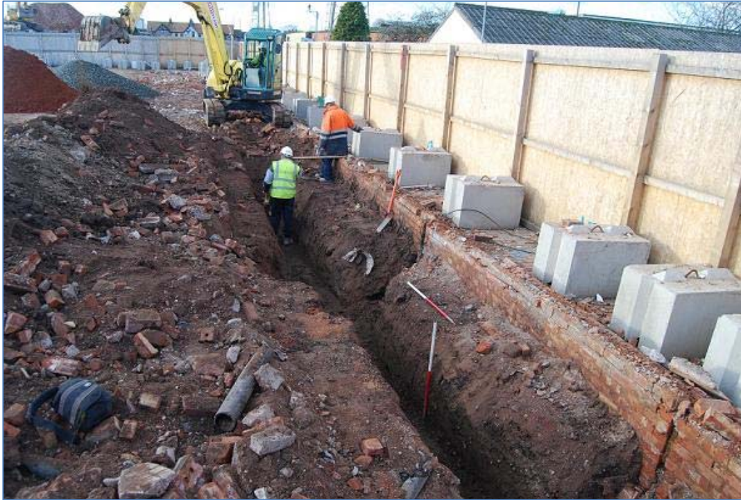
Plate 1 HV cable west of entrance. View northwest.
