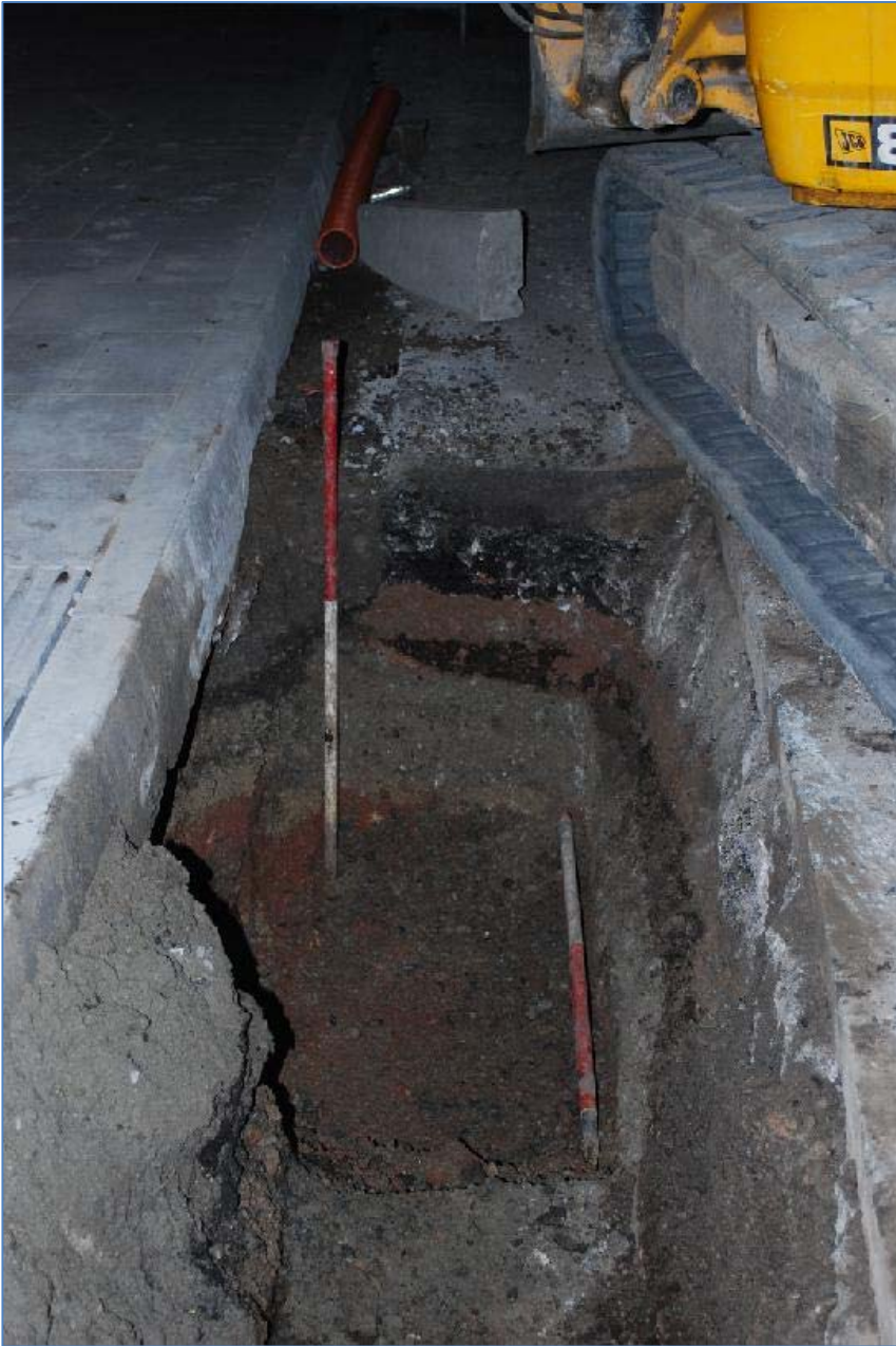
Plate 17 Gully pit adjacent to Wall Street showing layers of road make up and very compacted red gravel. View west.
