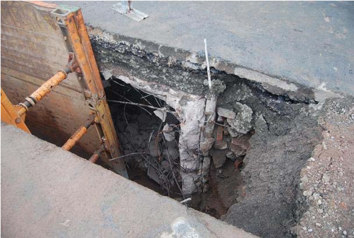
Plate 4 part of the modern subway under the road made of reinforced concrete.
