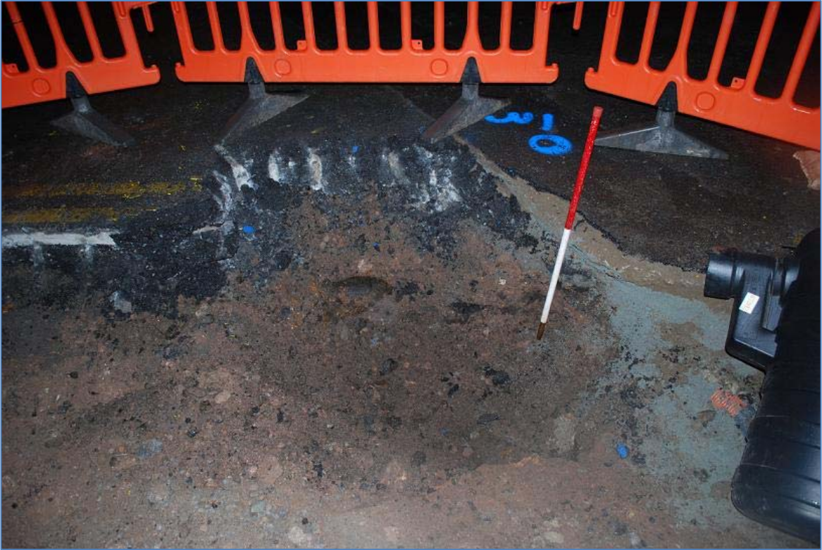
Plate 18 Widemarsh Street Gully Pit, showing modern water main and backfill of modern service trench. View West.
