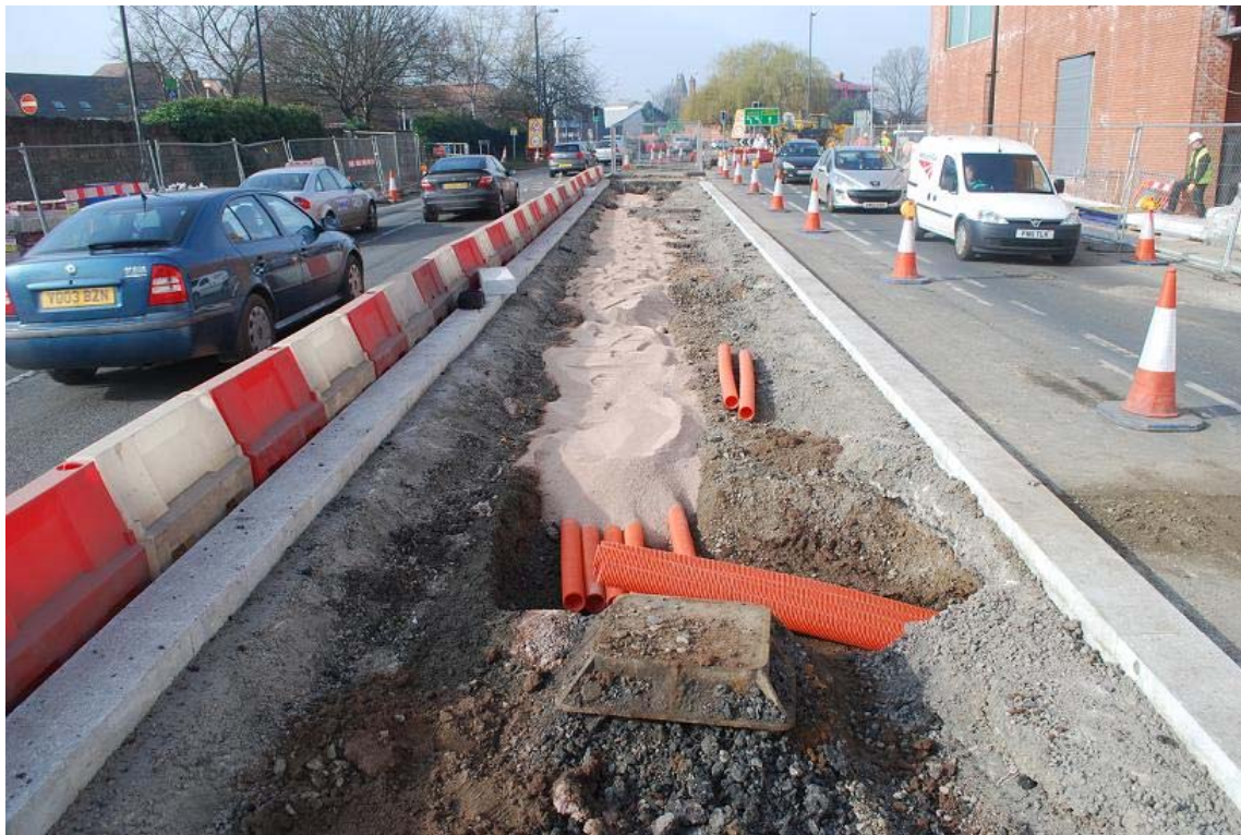
Plate 8 Example depth of ducting in central reservation and across carriageways after installation and backfilling.
