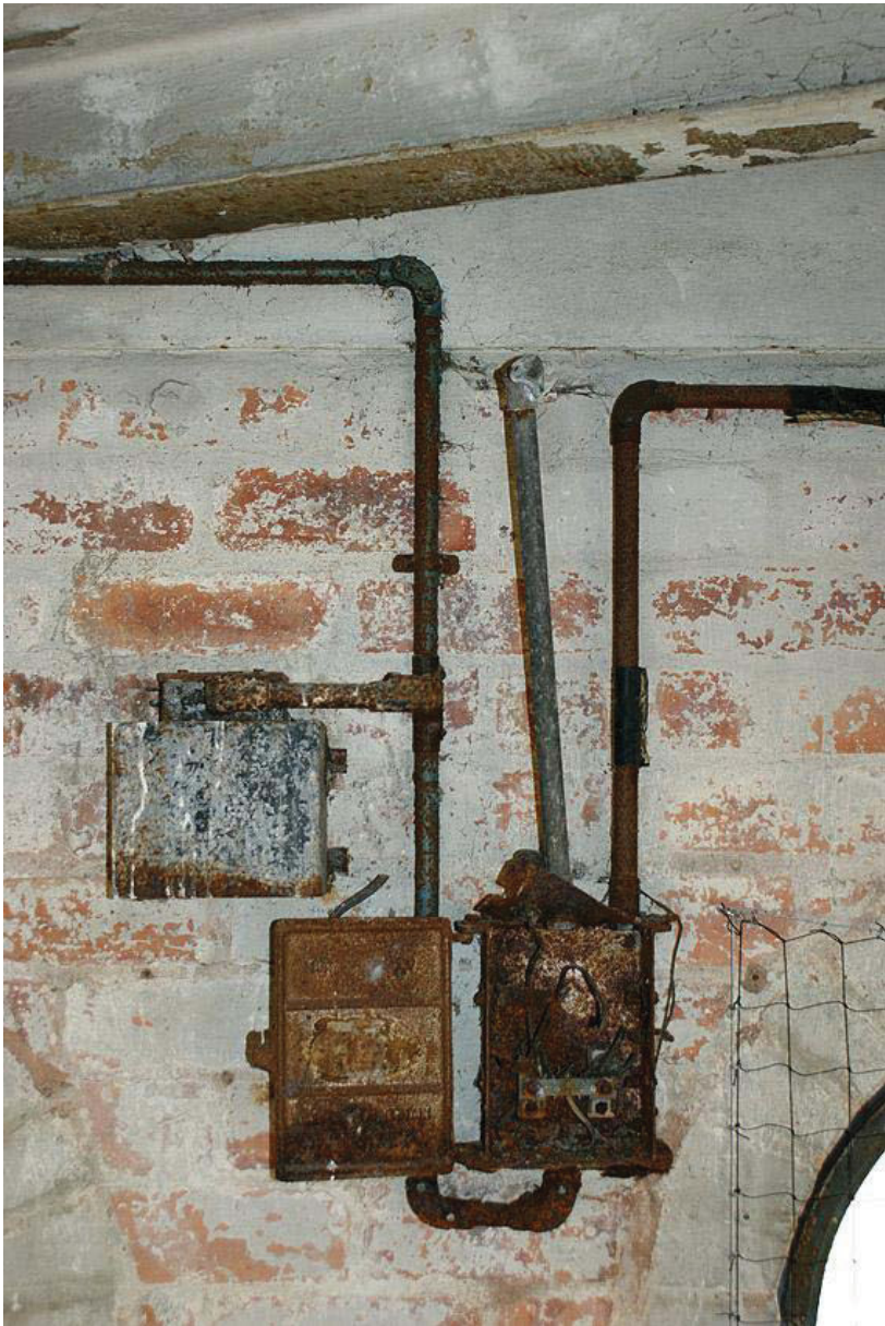
Plate 27: Original electrics within tower
