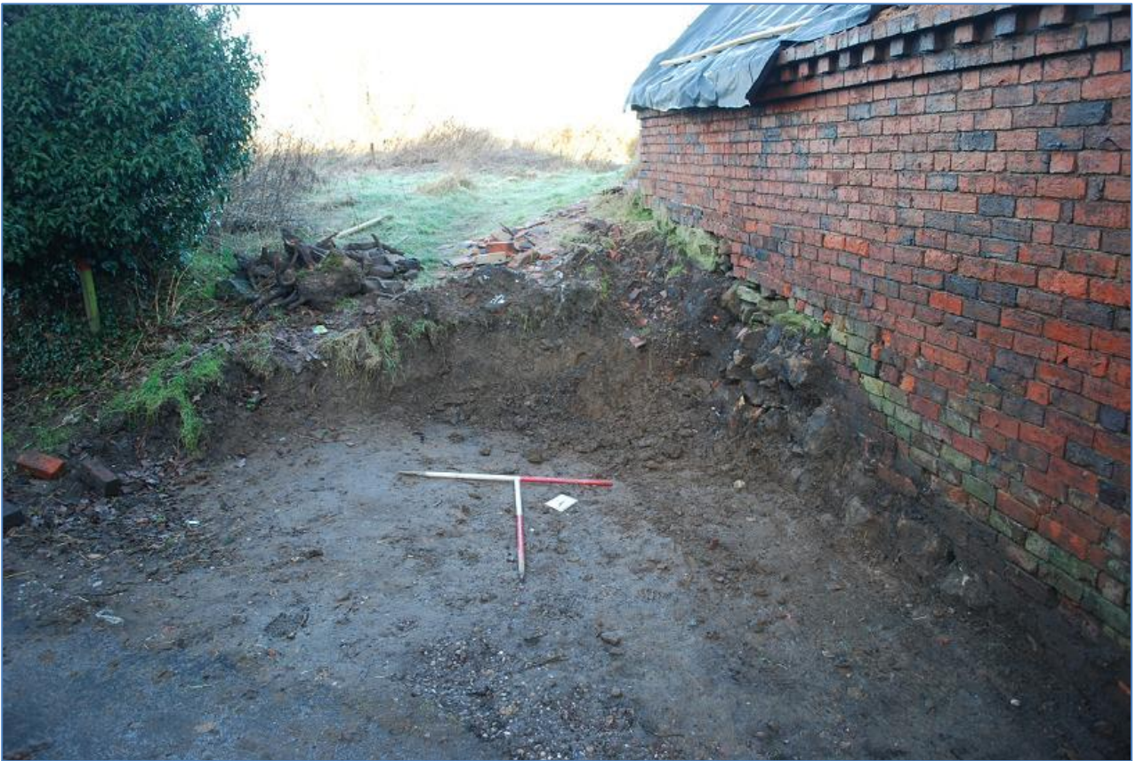
Plate 5 Bank to the south-west of barn reduced for car park. View north
