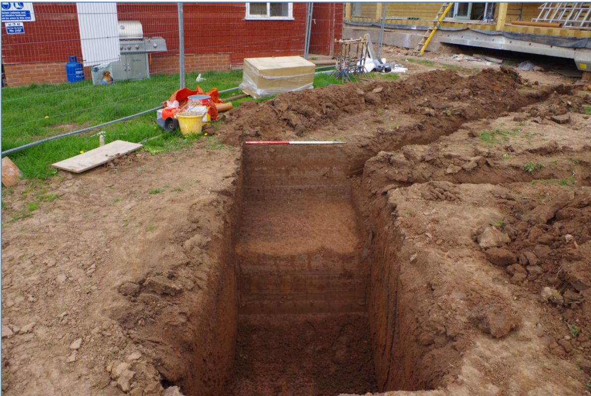
Plate 13: Trench 9 soakaway trench with pit 904 in north-west corner, view north, 1m scale
