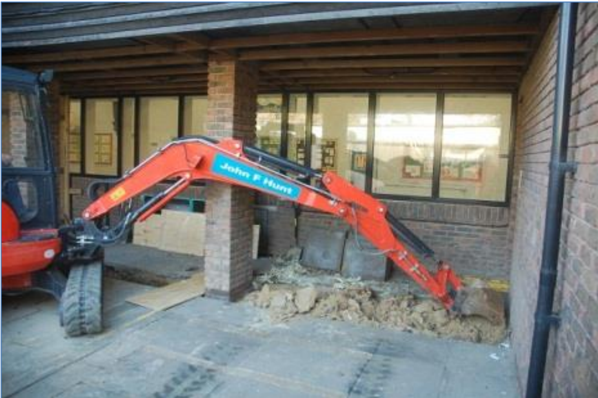
Plate 7 Location shot of Trench 4 ground beam excavation at school hall entrance in progress
