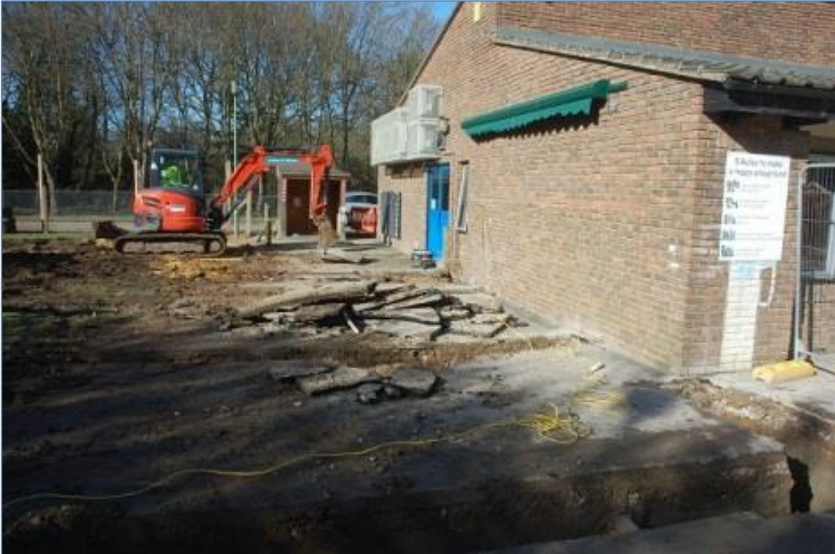
Plate 5 Location shot of Trench 3 ground beam excavation for the south-western extension in progress
