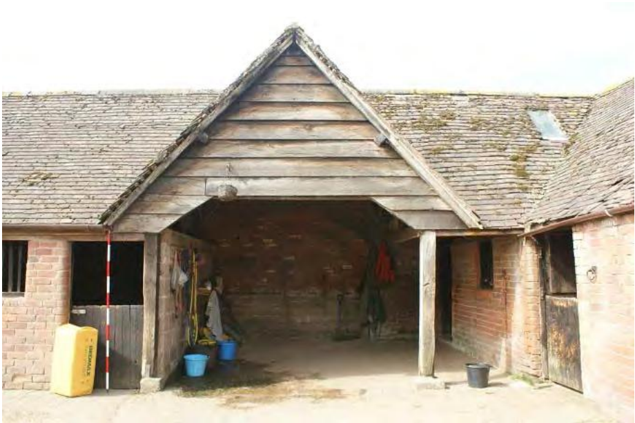
Plate 2 Blocked cart entrance, looking west
