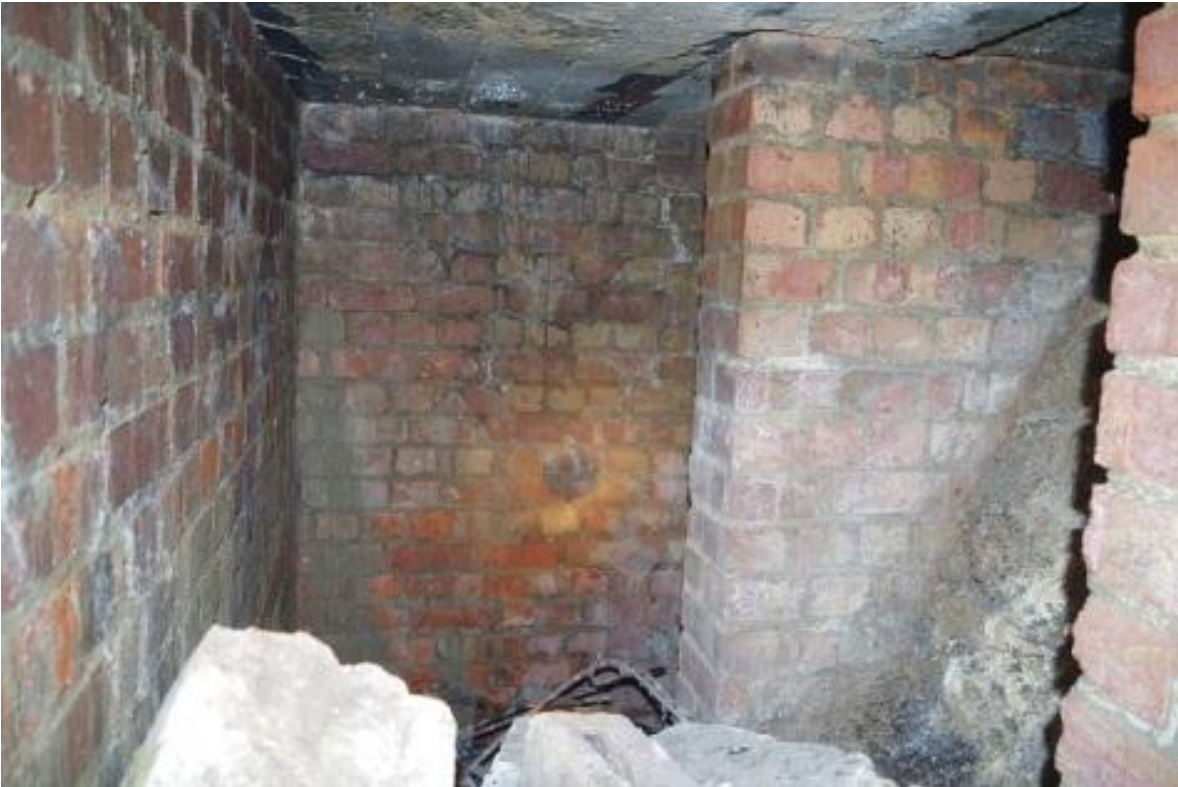
Plate 12, Interior view of the west end of the corridor on the southern side, and blocked west entrance, looking west
