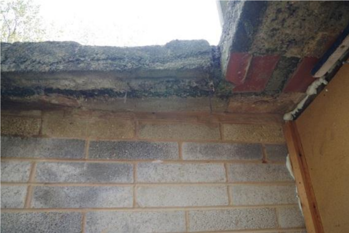
Plate 15, Exterior detail of later breeze block wall and former east entrance lintel to south side of existing entrance, looking south
