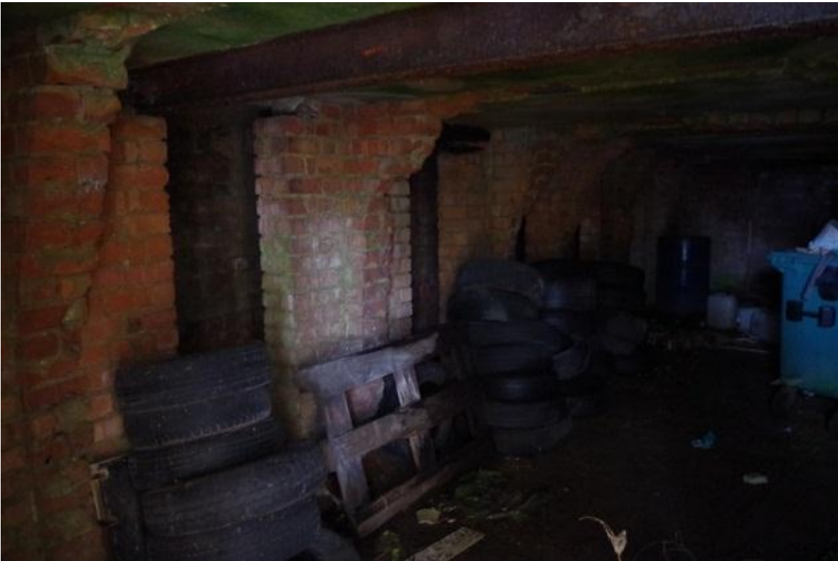
Plate 7, Interior showing the truncated wall divides, the doorways to southern corridor, and inserted cast iron joist, looking south-west
