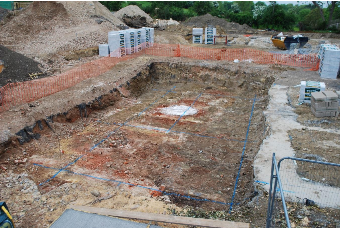
Plate 6 The two limekilns in Trench 5 after reducing to the depth of the required footings; view west
