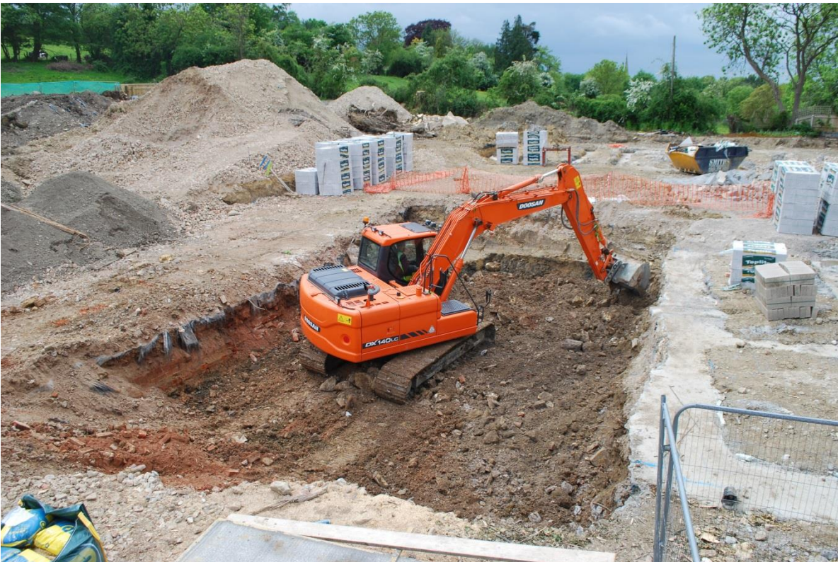
Plate 12 Trench 5 after removing the limekiln pot foundations and surrounding walls; view west
