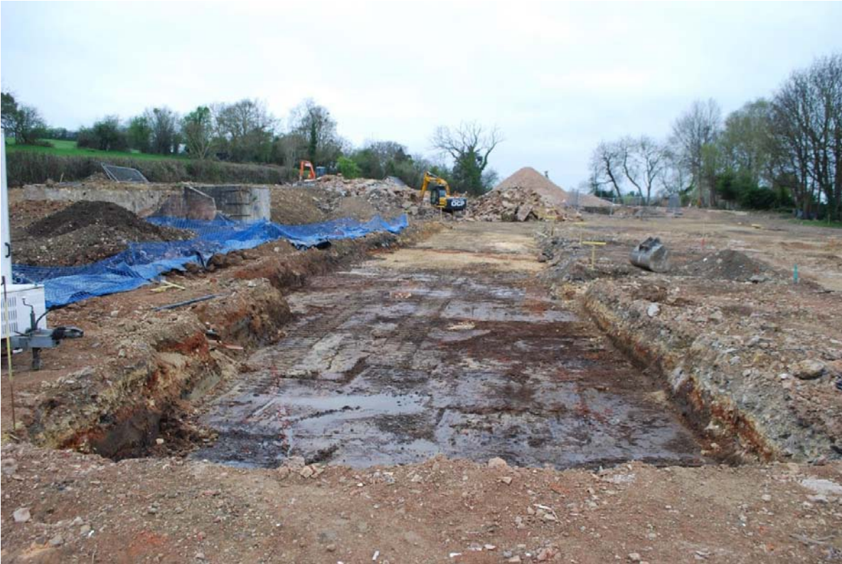
Plate 1 General view west of ground reduction (Trench 1), demonstrating the depth of modern made ground
