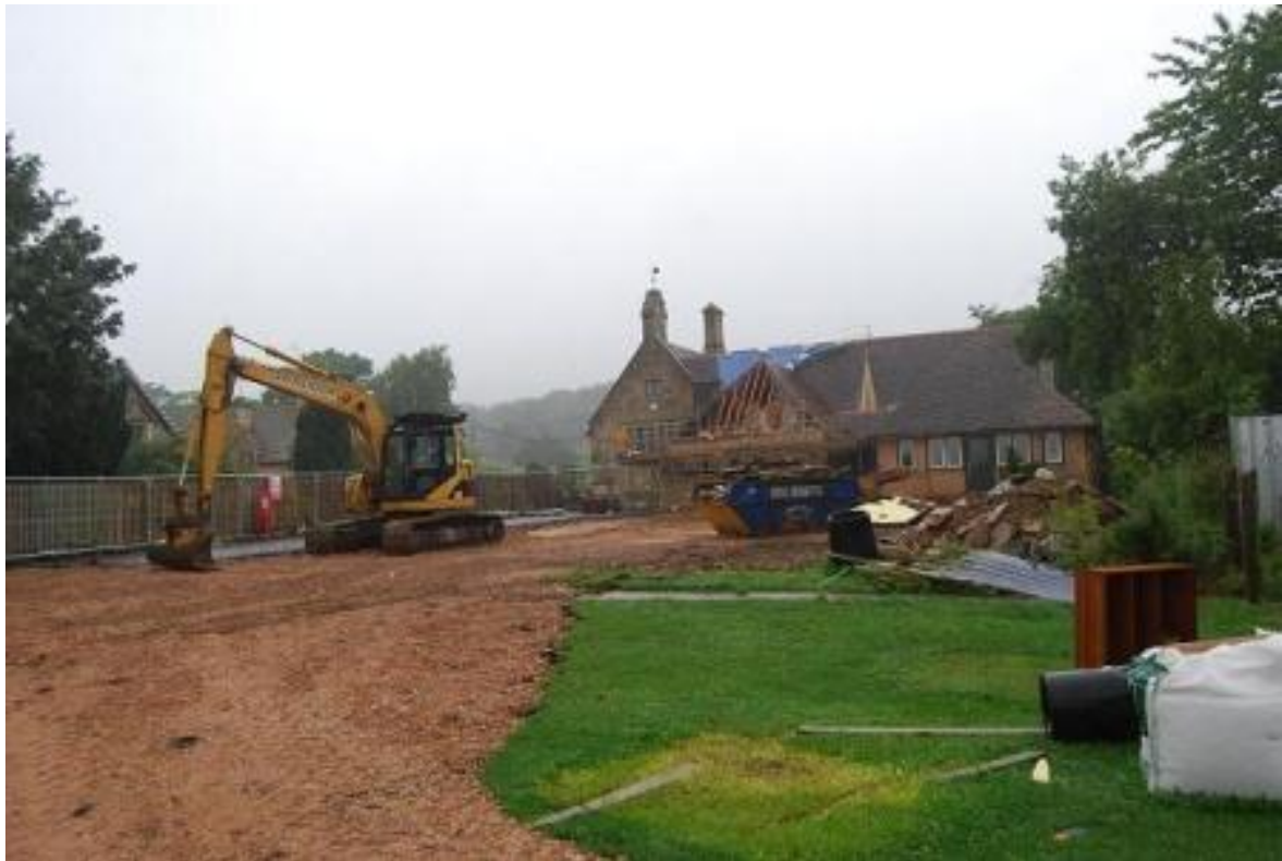
Plate 1: View of the development site during the first stage of work, facing north-west
