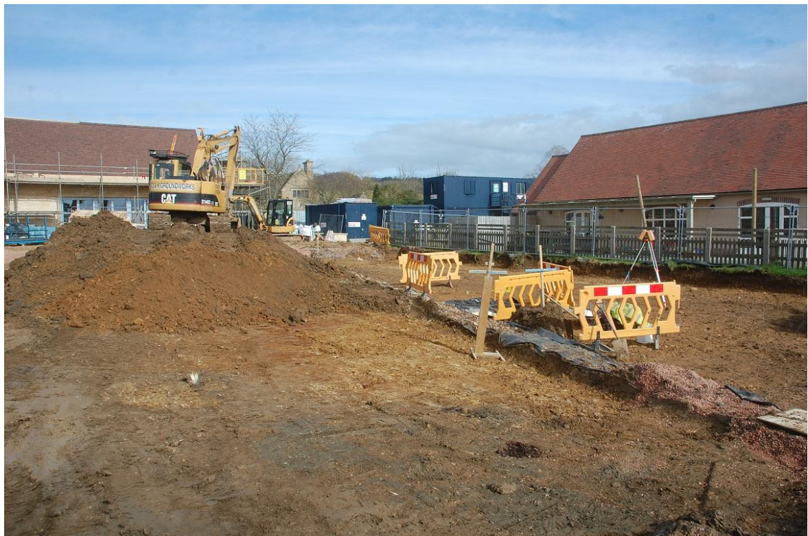
Plate 2: View of the development during the second stage of work, facing north-east
