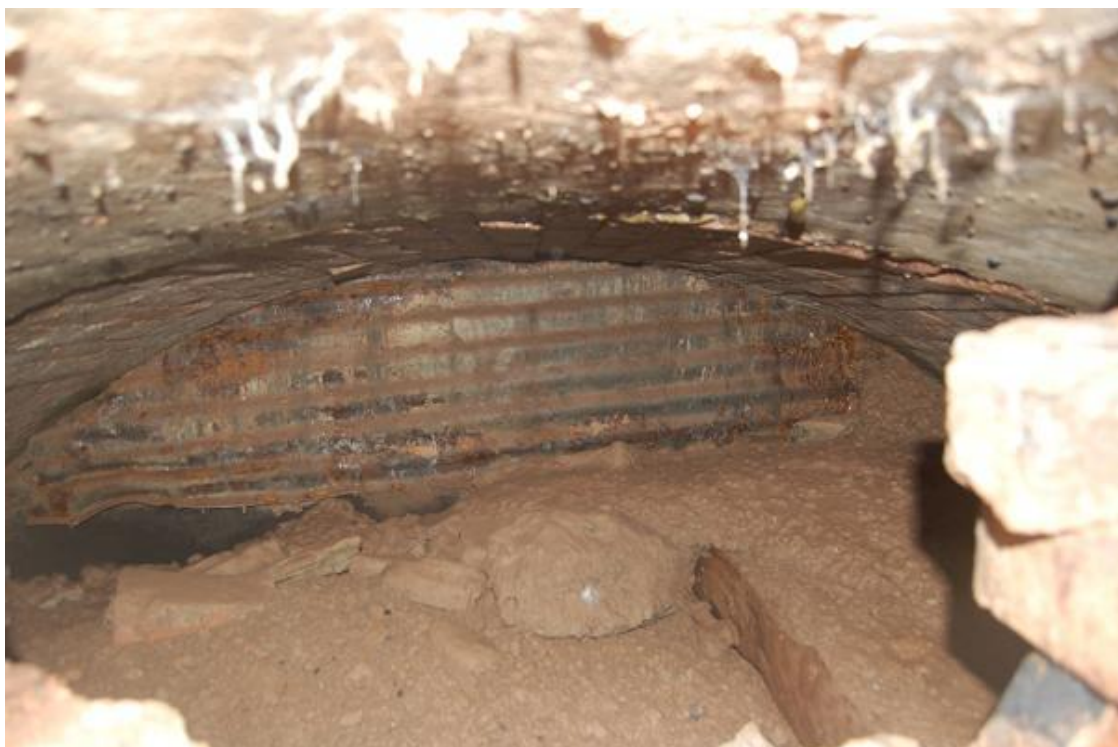
Plate 26 Internal void in Access Hole 1 (Trench 13), view west showing concrete and brick arches and earlier sandstone block wall to rear
