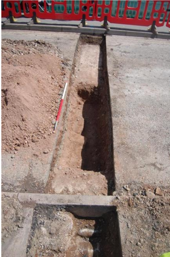
Plate 9 Span 4 (Trench 7) looking east at the existing sandstone bridge and concrete extensions
