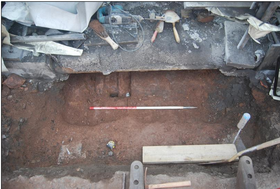
Plate 8 Excavation down to the keystones to be replaced through the original bridge in trench 1
