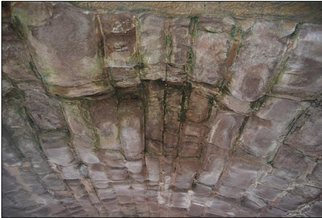
Plate 5 Damage to bridge keystones under span 6
