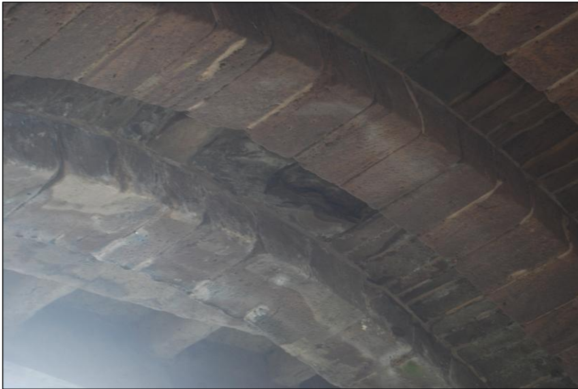
Plate 11 Damage to keystones under span 2
