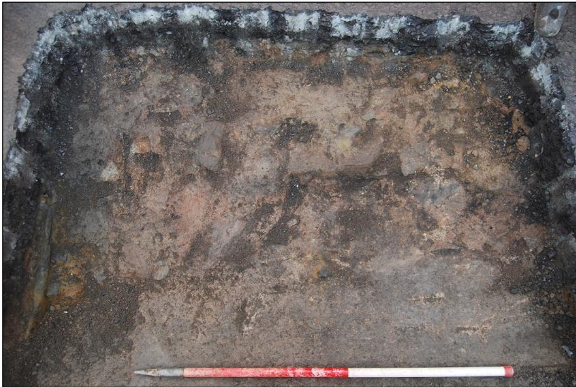
Plate 13 Trench 2 showing original road surface and overlaying modern tarmac road. The metal bars spanning the concrete extension and the original bridge can be seen in the bottom left corner of the photograph
