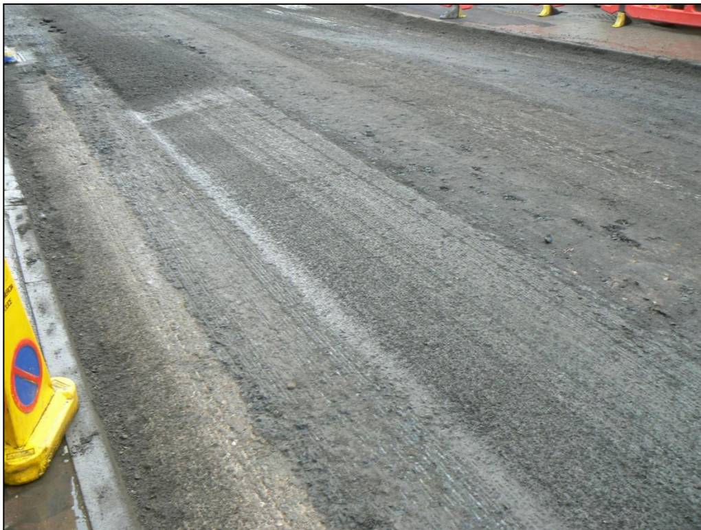
Plate 4 Centre of carriageway tarmac with 0.95mm planed off to reveal sound road base (courtesy of Richard Attwood, Worcestershire Highways Agency)
