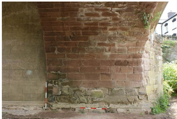
Plate 5: Interior of span 5, showing erosion on right, from the north
