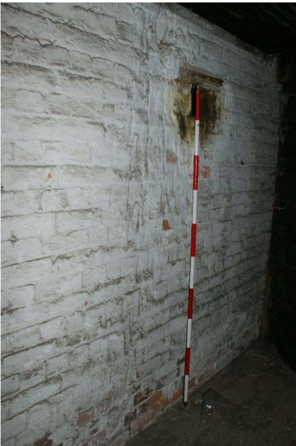
Plate 12 Wear on an internal wall showing the position of a former winch, looking north-west
