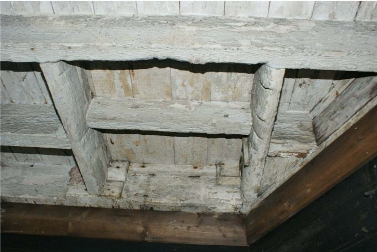
Plate 13 Gap in the floor joists for an internal winch hatch on the third floor
