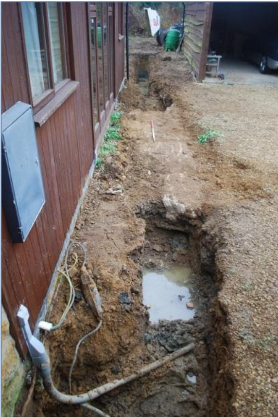
Plate 4 Trench 2 view southeast showing concrete hard standing block and service trench for electric, BT and water connections.
