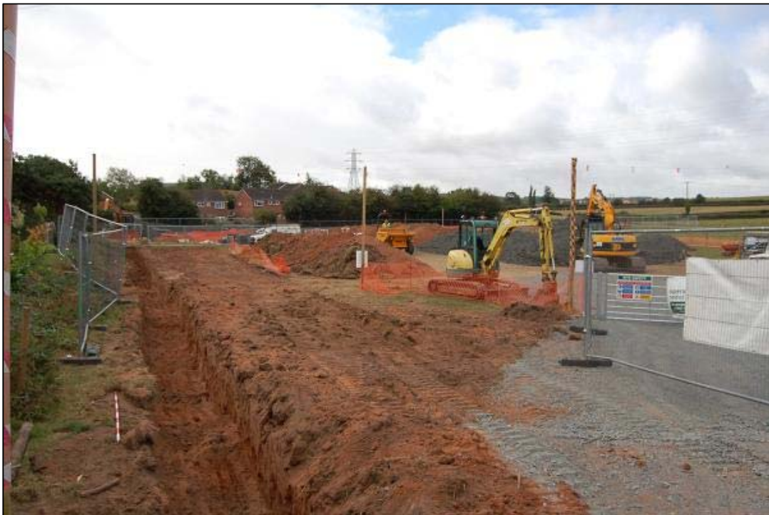
Plate 12 General shot of site showing Trench 4 excavated looking south and clay pile for creating the bank
