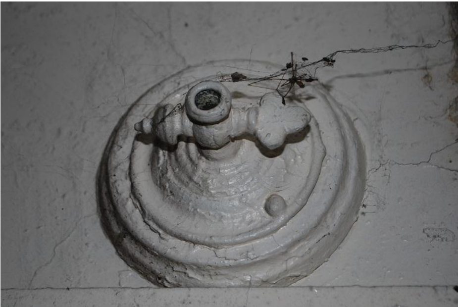
Plate 38 Detail of a gas light fitting
