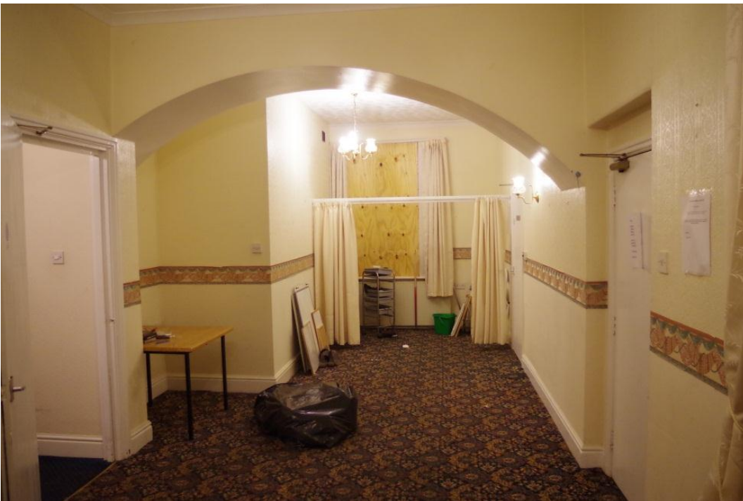
Plate 48 Ground floor of the service wing with the central wall removed, looking south west
