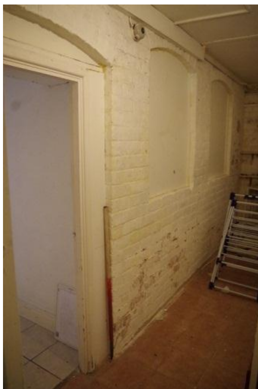
Plate 30 Blocked windows into the coal cellar looking north east
