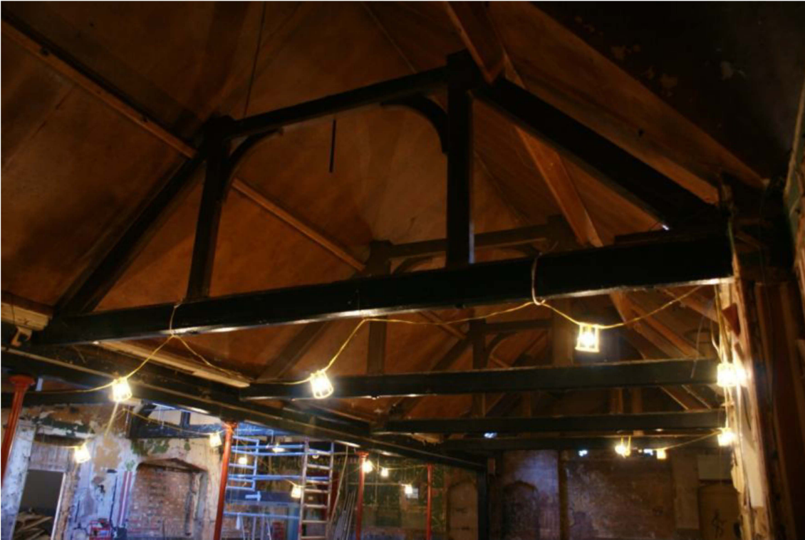
Plate 13: The roof structure of the former school building with tie beams and queen post trusses.
