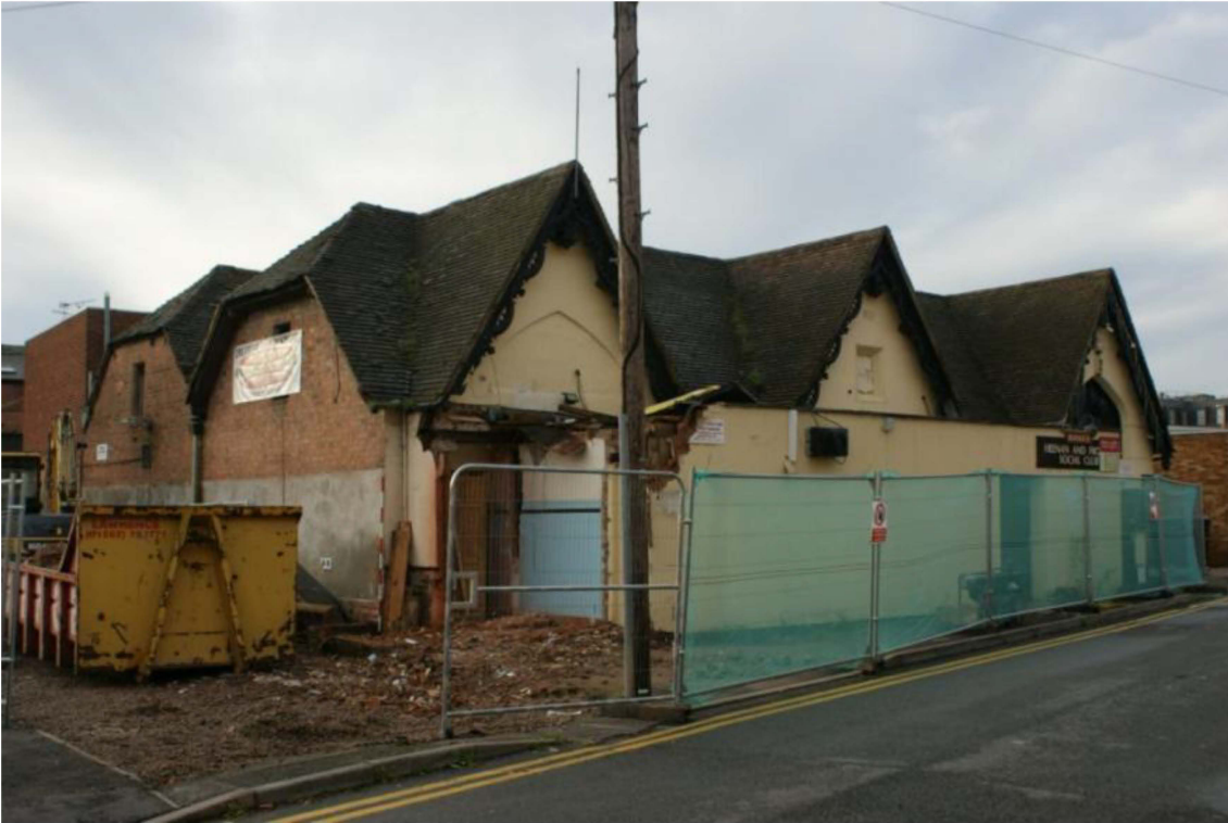
Plate 7: The former school and social club building with a 20 th century extension
