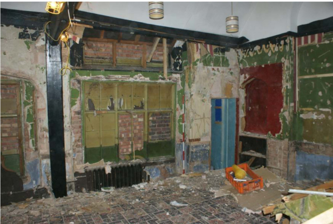
Plate 14: A blocked former window at the rear of the former school building.
