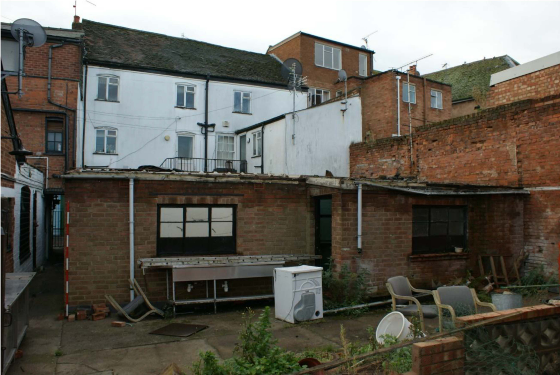
Plate 27: The flat roofed building at the southern end of the plot, built between 1940 and 1965.
