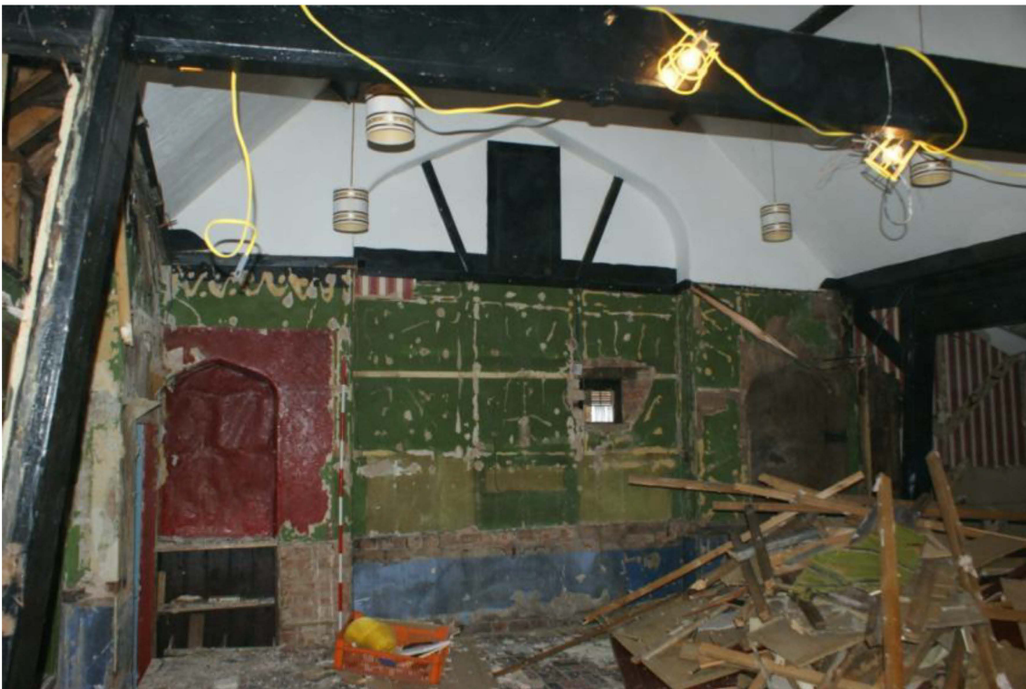
Plate 10: Architectural interior detailing within the former school building with a former blocked window within the central arch.
