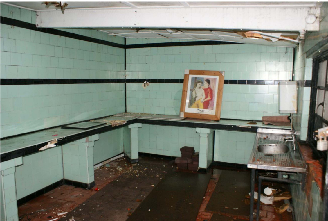
Plate 28: Kitchen contained within the flat roofed building at the southern end of the plot.
