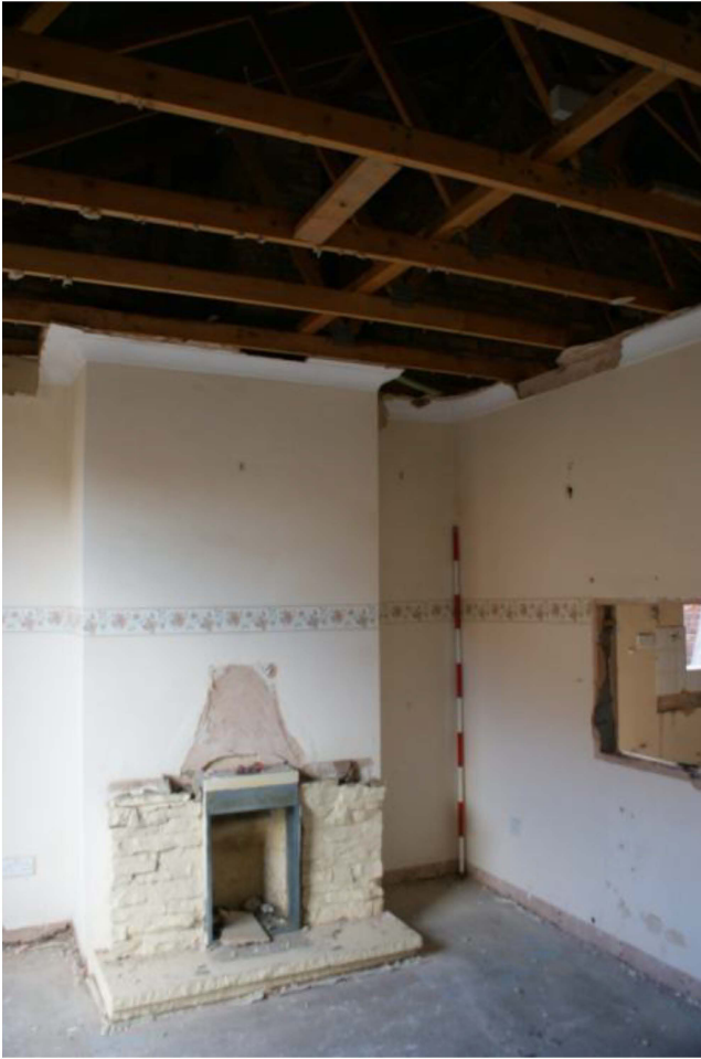
Plate 21: Interior of the bungalow showing the modern replacement roof timbers and the modern breeze block interior walls.
