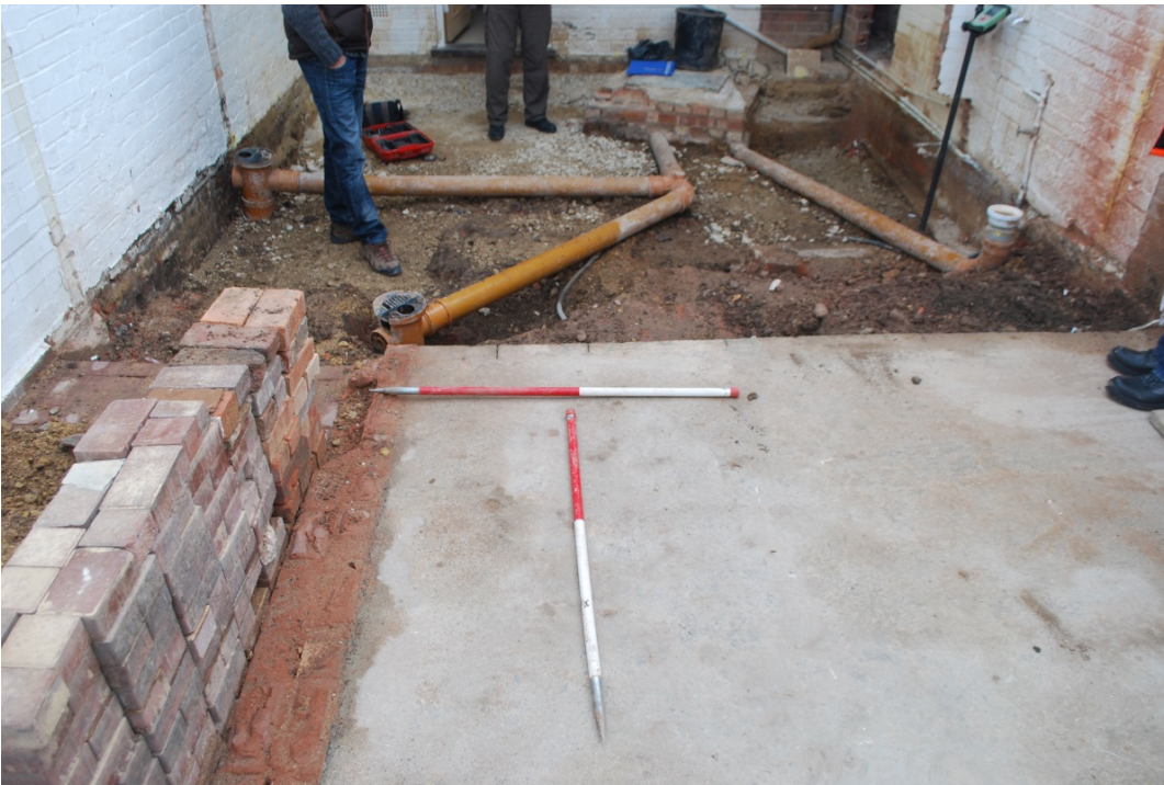
Plate 2 The concrete floor overlying the cellar and modern drainage, looking east (1m scales)
