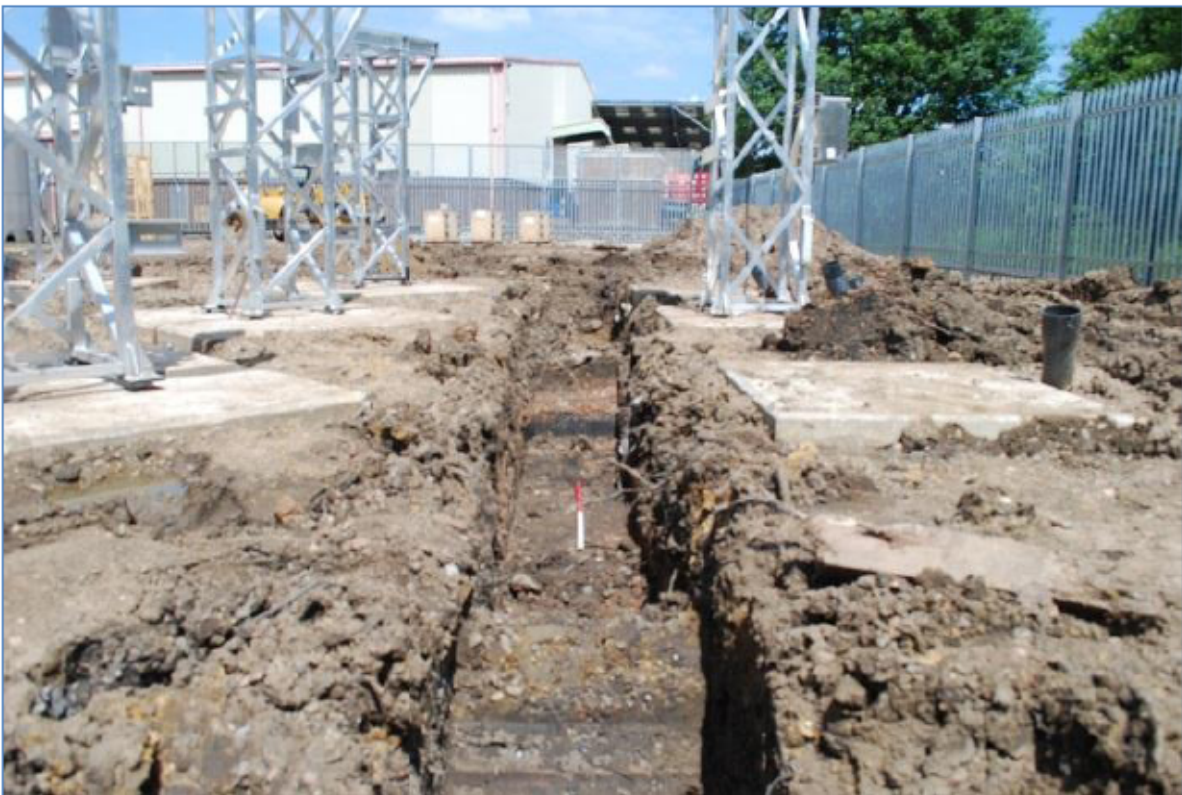
Plate 2 The trench between the substation structures; 0.50m wide and 0.50m deep to avoid structures; facing north
