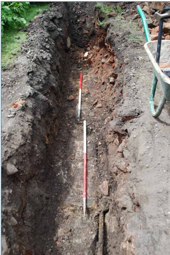
Plate 6 The sandstone slab causeway (708) in situ with water pipe trench to north; view west
