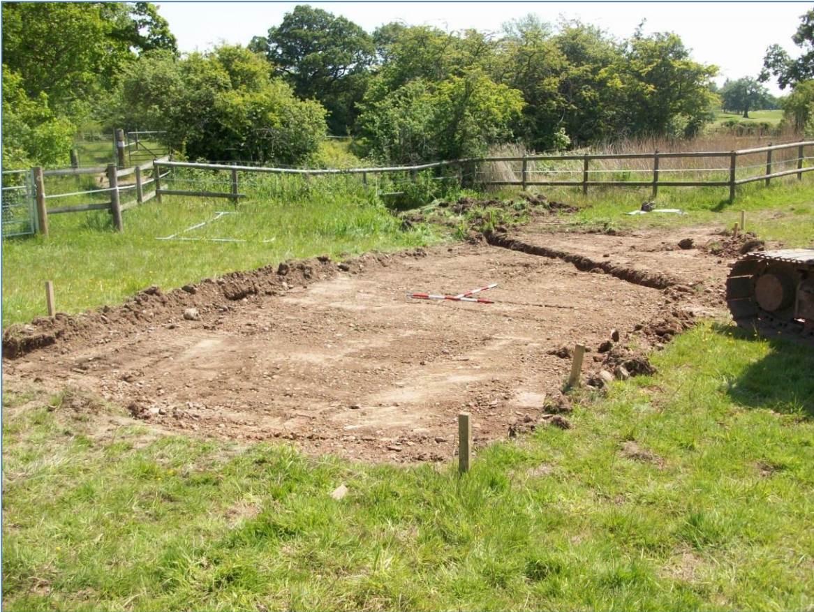
Plate 1 Trench 2, the area for the reed bed stripped of topsoil; view south-east
