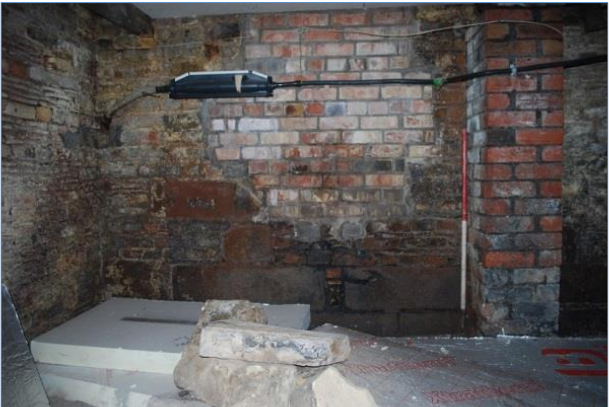
Plate 10 Blocked up coal chute on southwest side of cellar, showing brick tile and sandstone construction and modern additions. View south.
