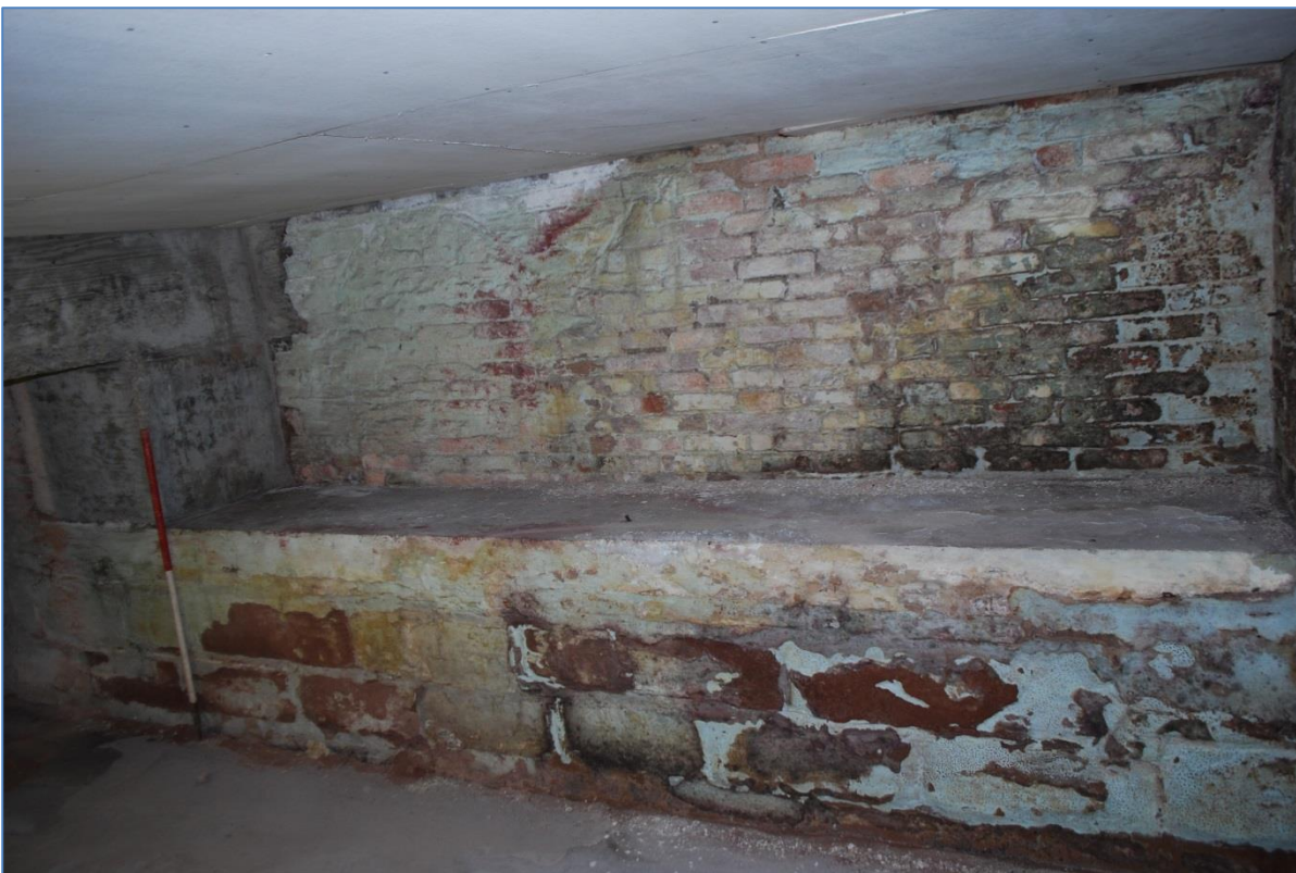
Plate 12 Shelf for stored beer barrels on eastern side of cellar. View northeast.
