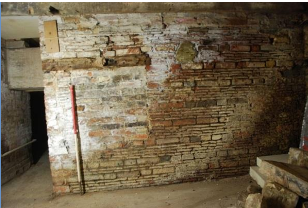
Plate 6 Brick and tile wall of cellar showing later blocked up area and wooden beam. Passage between the two rooms is to the right of the photo, with the modern concrete beams also evident.
