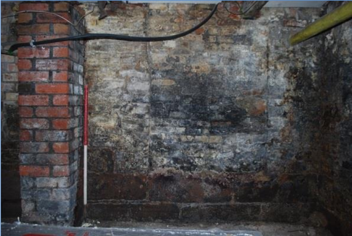
Plate 11 Second blocked up coal chute on southwest side of cellar. View south.
