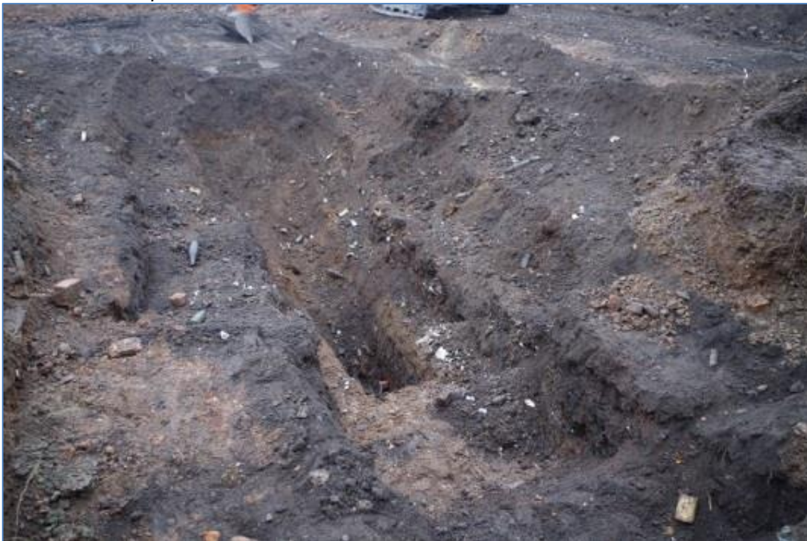
Plate 2 Evaluation trench 1 showing unstable nature of made ground and stepping
