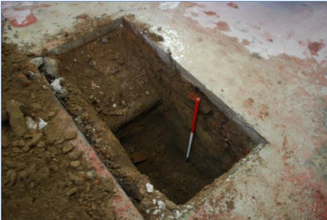
Plate 9 Geotechnical pit 18 (TP201) showing cast iron pipe and natural strata within garage.
