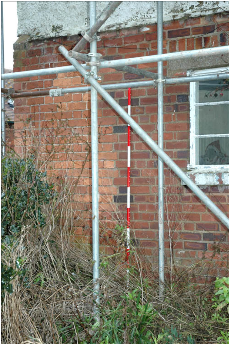
Plate 32: 20 th century repair building break on south elevation
