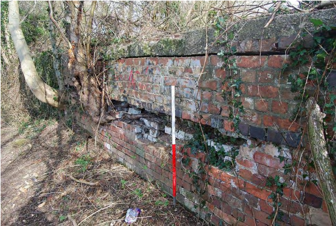
Plate 1 Part of the brick wall forming the eastern boundary of the development site, thought to relate to Harborne Mill
