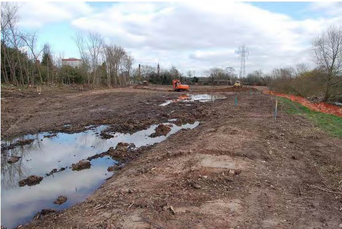
Plate 7 Existing soil bund running along the southern edge of the reservoir, facing East
