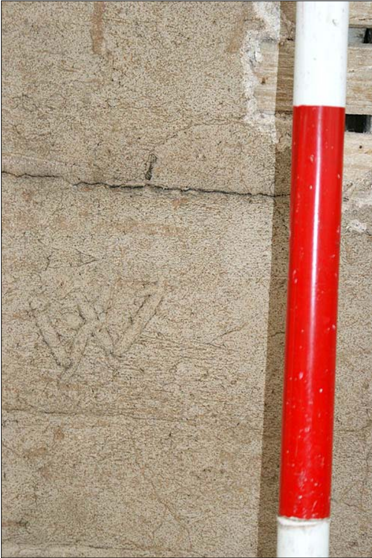
Plate 25: Intersected Vs on attic 1A partition
