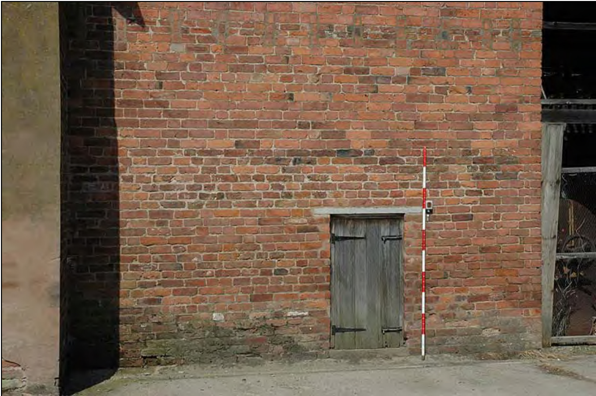
Plate 2: 17 th century wall now part of east wall of the hop kilns
