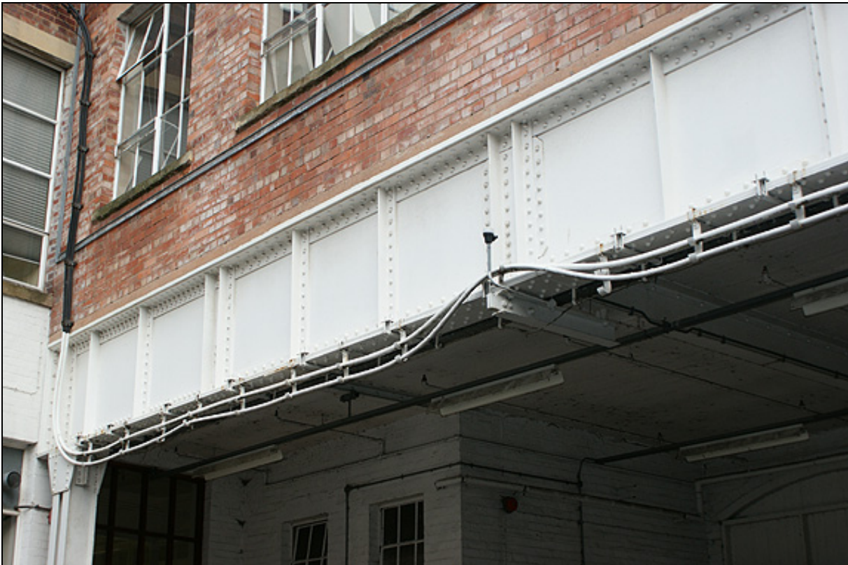
Plate 41: Massive RSJ 'T' beam in yard
