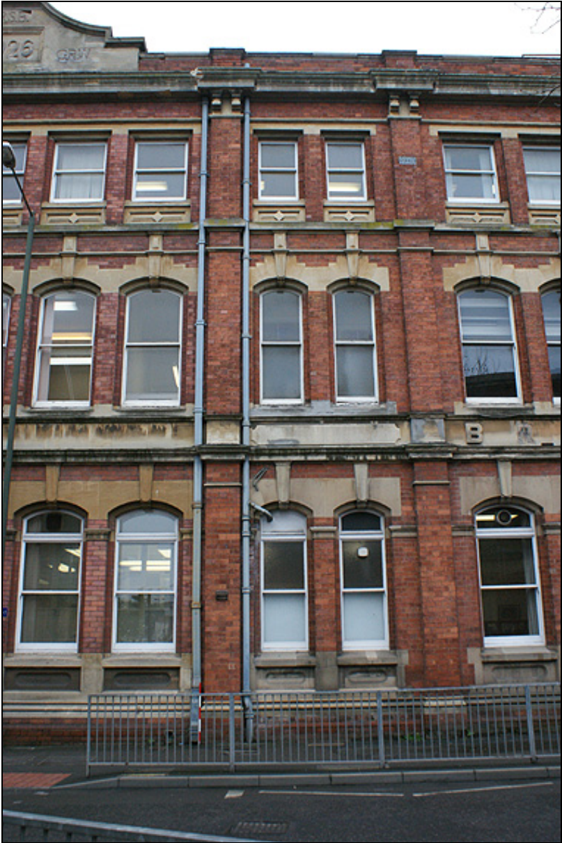
Plate 36: The same limestone detailing (left of the drainpipes is 1926, to the right is 1876).
