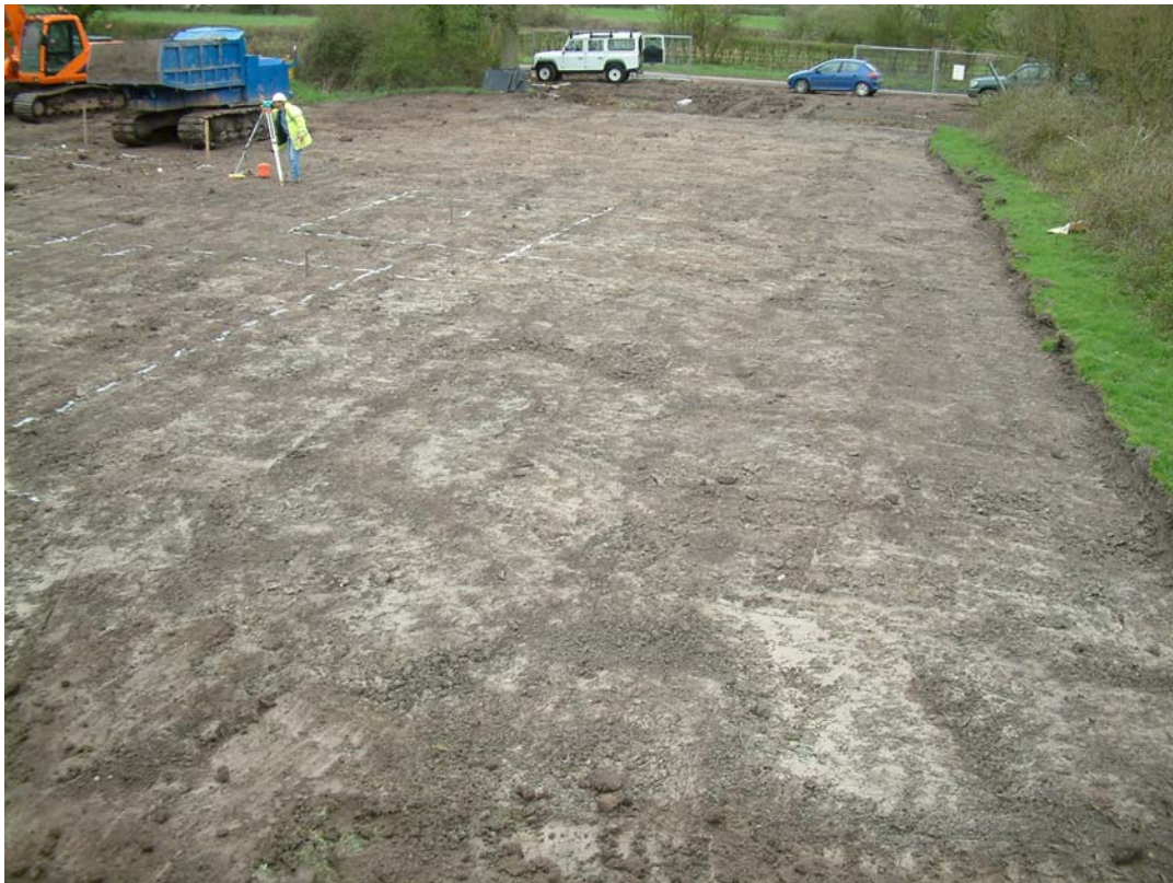
Plate 2: Stripped site with the location of the settling tanks being marked out, facing north
