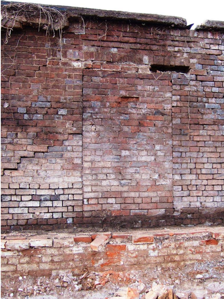
6. Blocked doorway in Mrs knight's garden wall, exposed after demolition of malthouse
