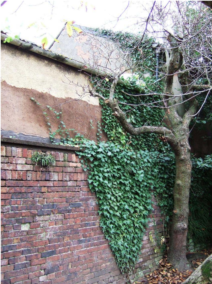
5. Detail of W. Elevation including garden wall at kiln end of malthouse
