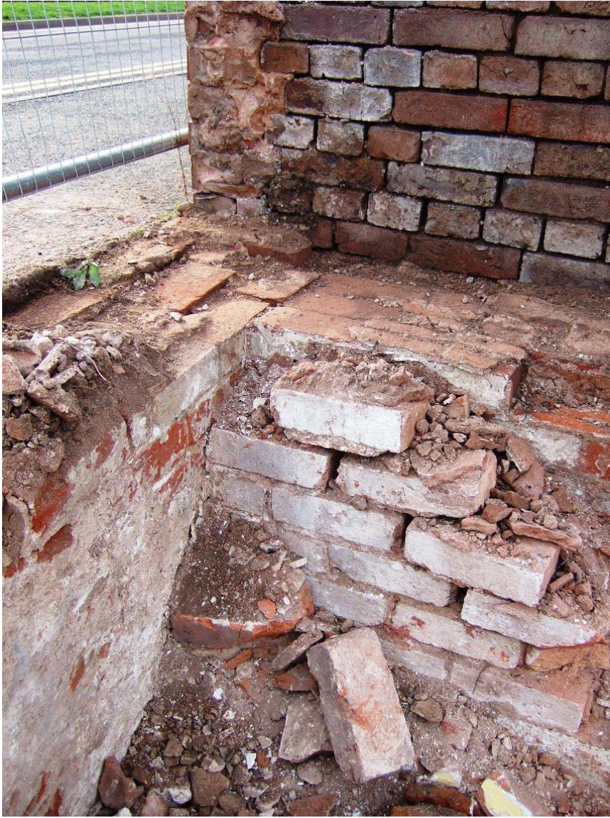
8. Detail of construction of S. Gable and W. Elevation basement walls, including later brick skim
