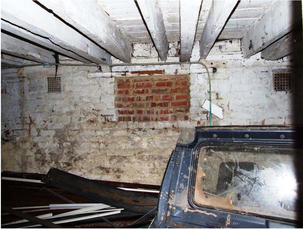
13. Basement E. Elevation, detail of blocked openings and floor joists, old and new
