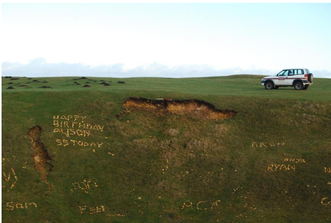
Plate 2: The area of erosion, looking north
