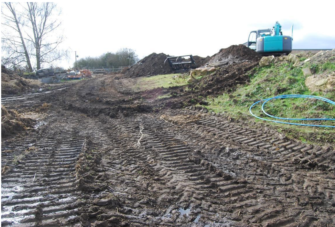
Plate 2, Location of the trench (to the far side of the excavator) showing build up of ground, view south-west
