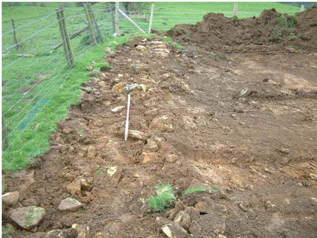
Plate 4: Collapsed dry-stone wall (103) between fields 2 and 3, facing northwest
