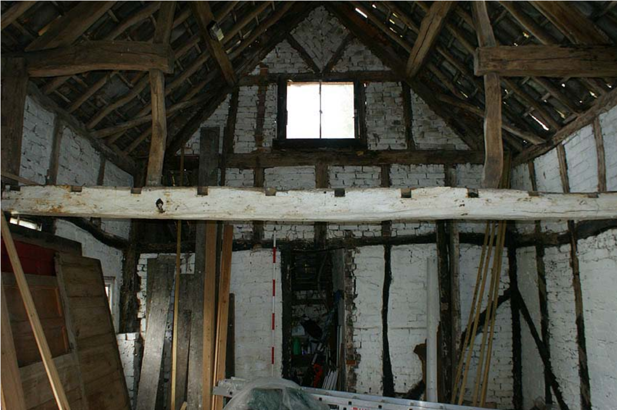
Plate 14: Truss 2, floor joist notches
