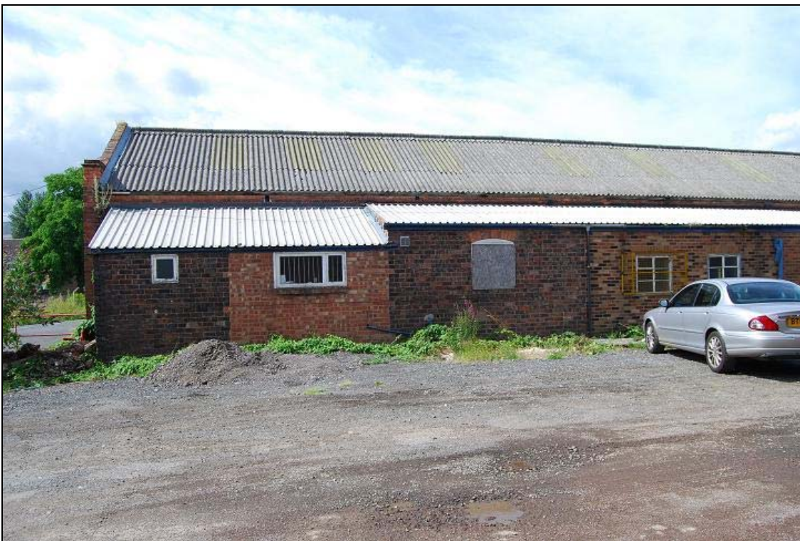
Plate 26: The north elevation showing the extension to the mid 20 th century building (Unit 25c).
