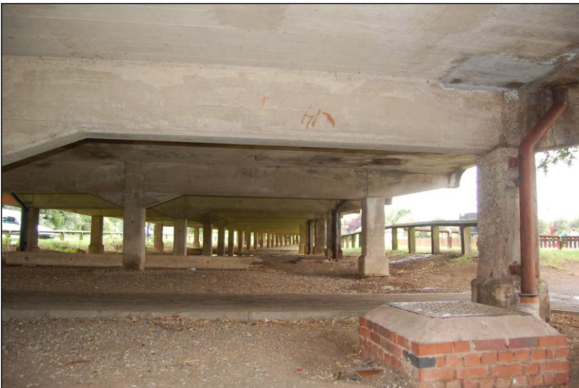
Plate 4: Piles and deck slab of the viaduct, view north from the north abutment of the bridge
