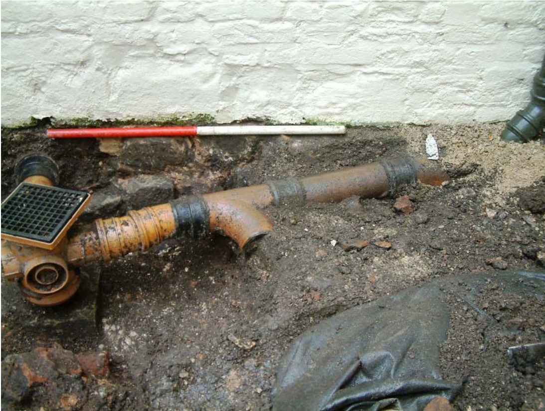
Plate 10 looking south: Test pit 3 showing existing modern drainage system with roof downpipe to upper right and surface drain to left. The pipe work runs through the Commandery House foundations (left of the photographic scale).
