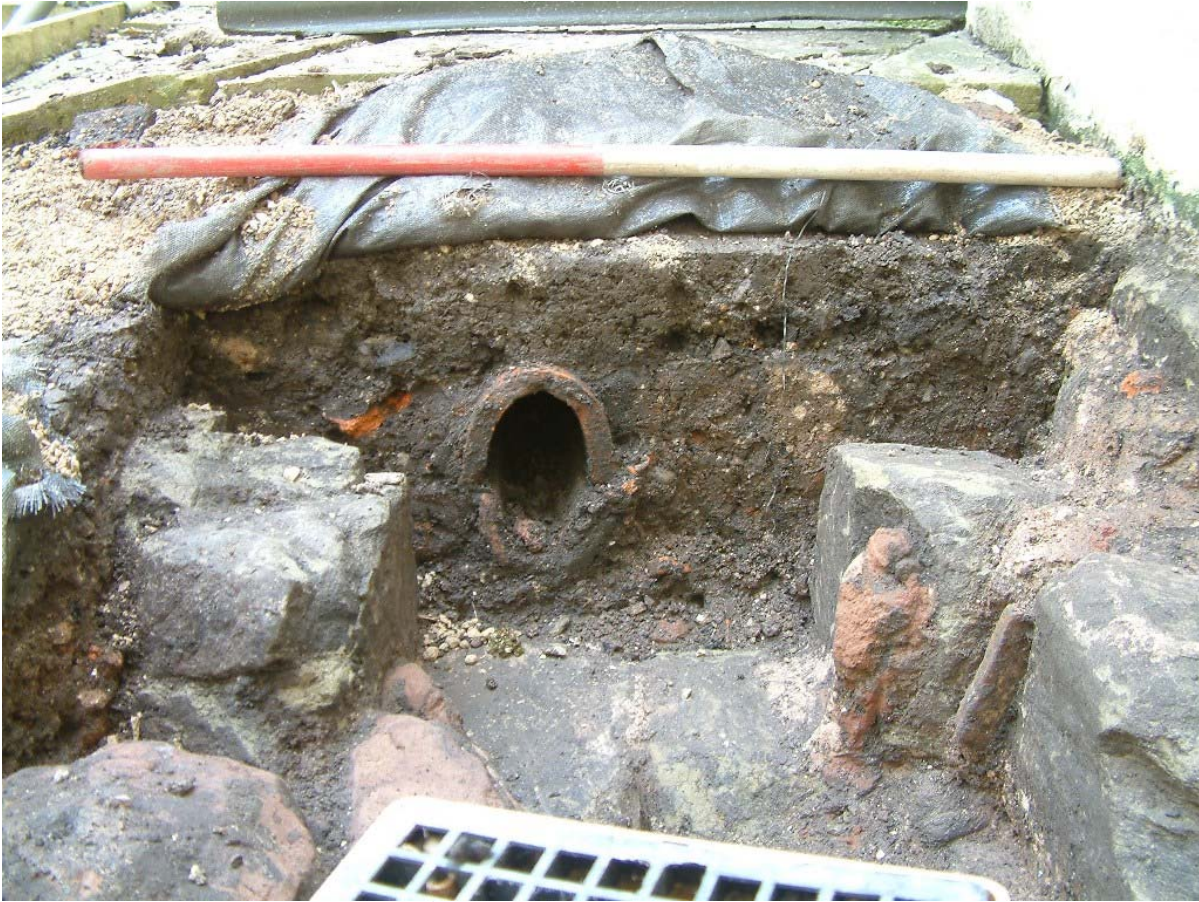
Plate 9 looking east: Test pit 3 with 19 th century drainage system and contemporary removal of chapel wall to accommodate pipe work. Existing modern surface drain in foreground.
