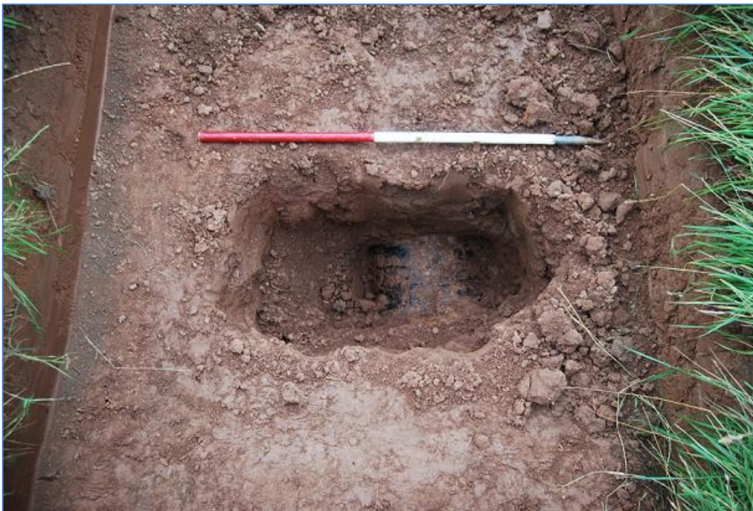
Plate 4 Close up of Trench 2 showing existing gas main at base, 1.00m below ground level; south bank of the River Teme
