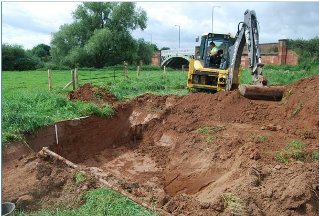
Plate 8 Trench 6 drilling egress pit looking south-west towards Powick New Bridge; north bank of the River Teme
