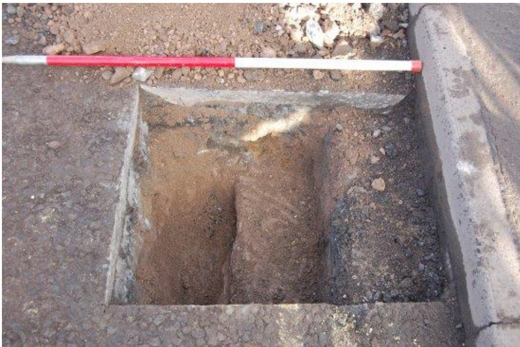
Plate 4: Test Pit 2, south facing section, prior to removal of modern concrete 103, scale at 1m (facing north).
