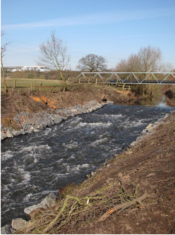
Plate 8 Severn Trent rising main crossing the River Stour; looking north-west. N.B – The completed Weir 2 is shown in the foreground.
