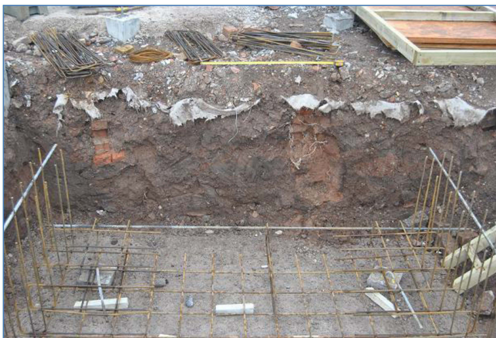
Plate 14 South-east facing section of lift shaft showing a series of soil horizons and modern levelling layers
