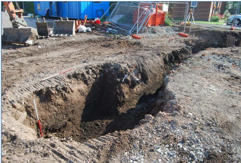
Plate 8 General shot of Trench 2 drainage showing series of modern made ground and levelling material, looking north
