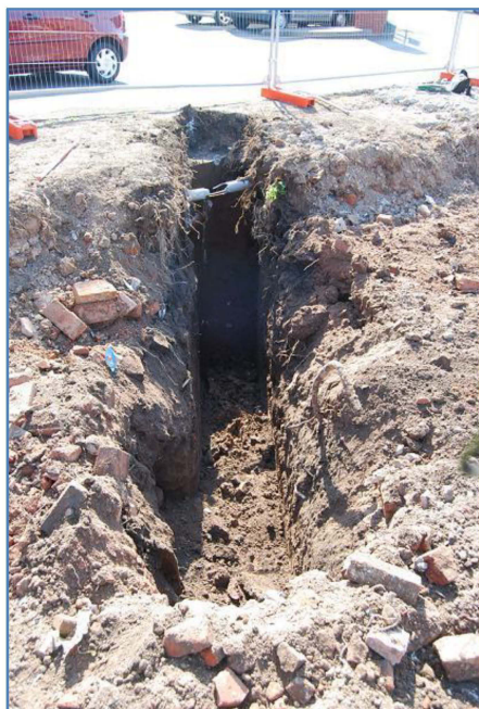
Plate 5 Trench 2 drainage connecting to existing manhole in east corner of site, showing manhole and BT cable at the back of the trench, view north-east.
