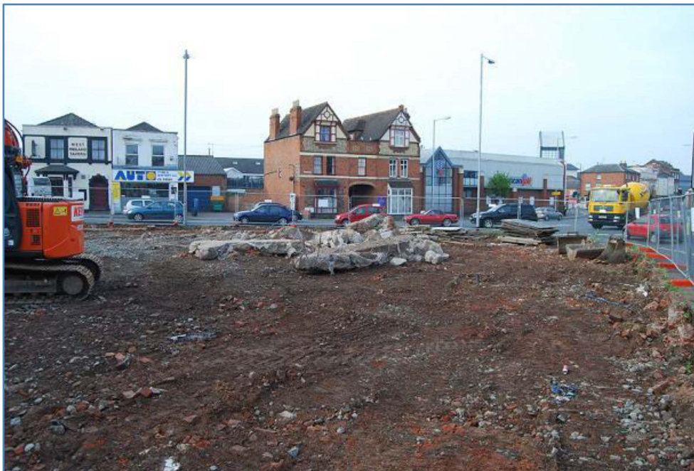
Plate 4 The reinforced concrete hard standing broken up across the site during the initial ground reductions, looking south
