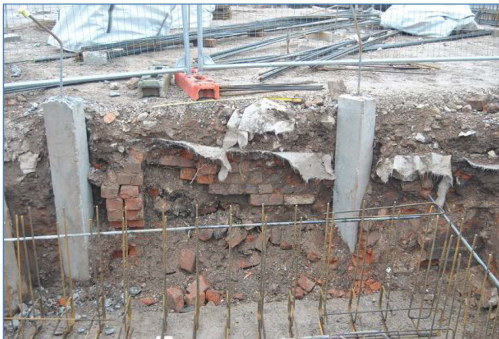
Plate 13 Lift shaft (Trench 3) north-west facing section showing cellars of previous building and modern piles for new development.
