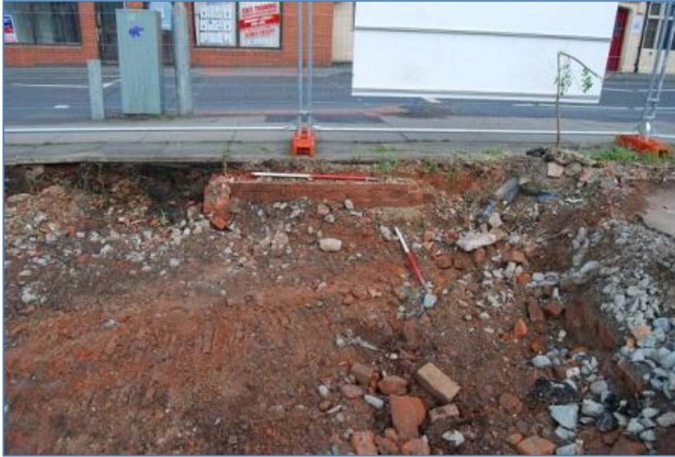
Plate 3 The final reduced depth in the north end of the site and a modern existing brick wall, looking northwest
