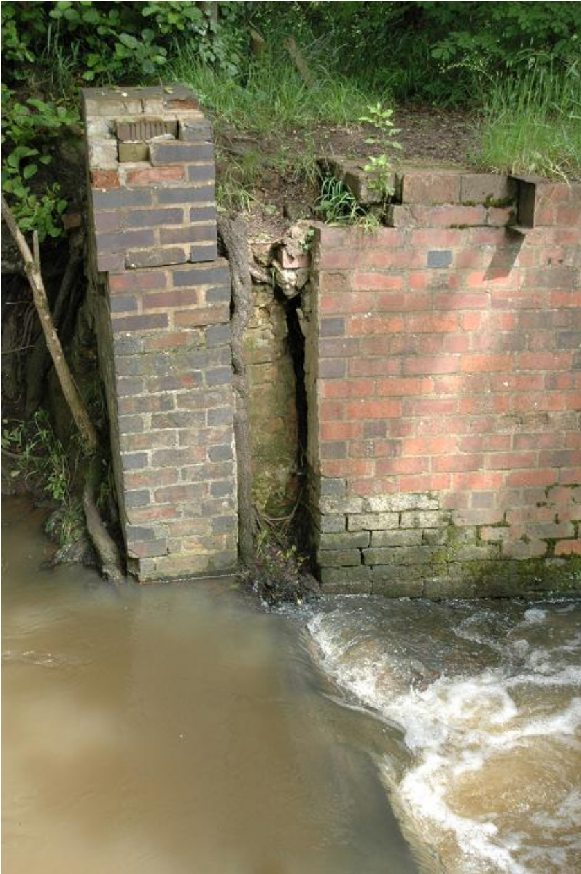
Plate 3 The housing for the old sluice, western side of Five Tunnels Weir, from the west
