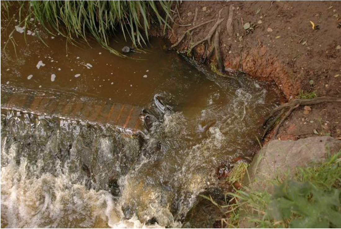
Plate 10 Erosion beyond the eastern edge of Five Tunnels Weir, looking north
