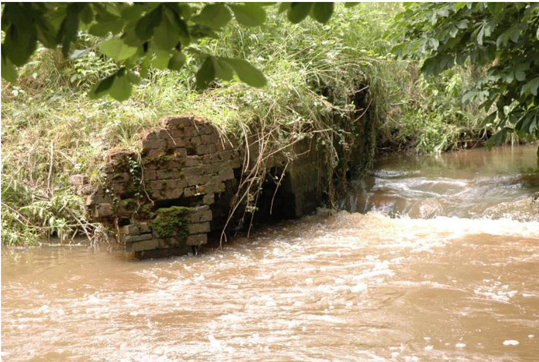
Plate 8 The western side of Mill Weir, in poor repair, from the east
