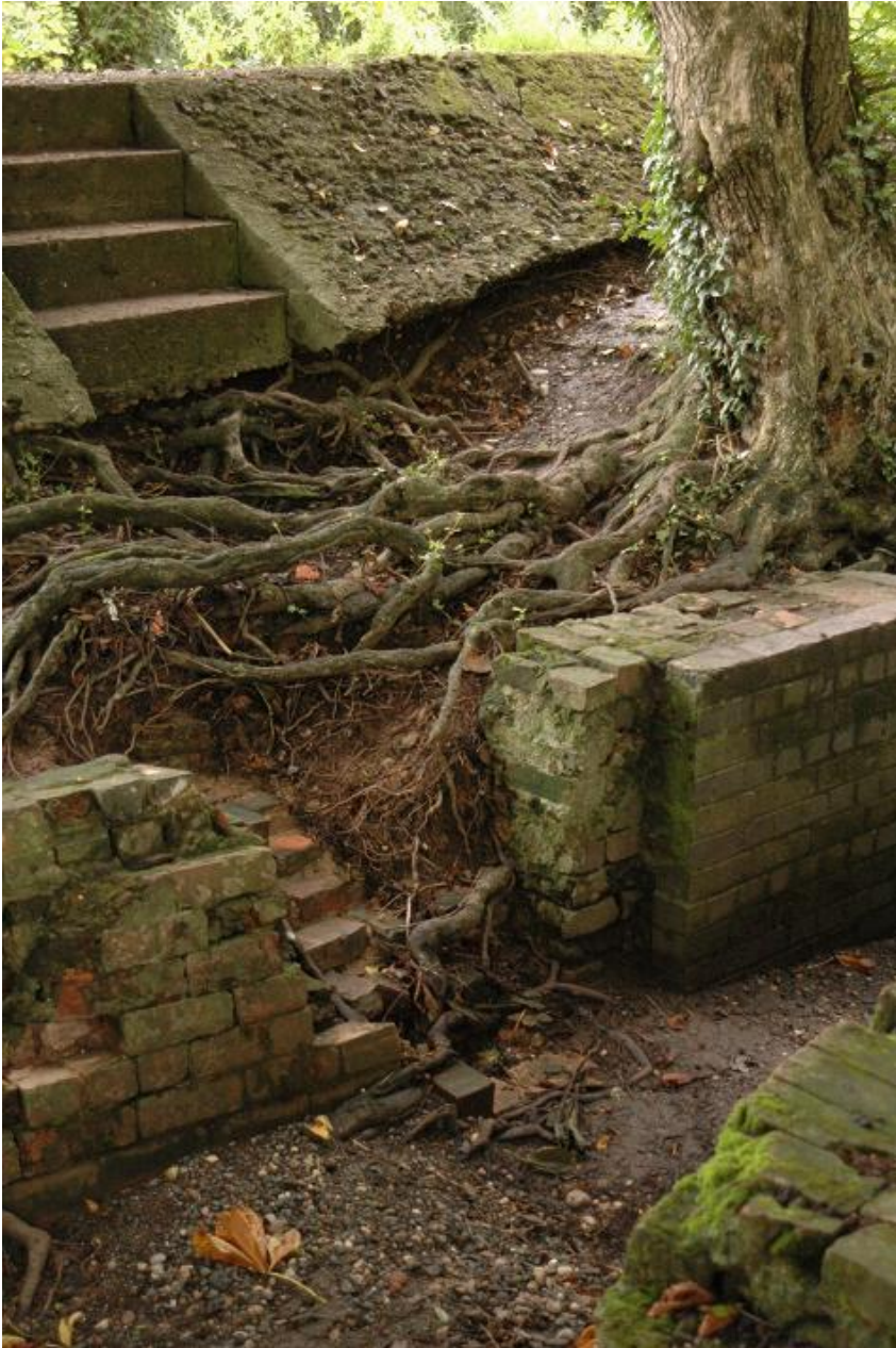
Plate 9 Tree root damage to the sluice remains by Mill Weir, looking south-east
