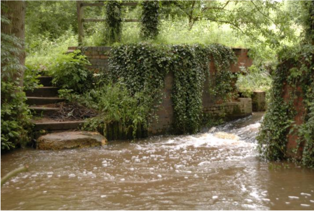
Plate 4 The western side of Five Tunnels Weir, in poor repair, from south-east
